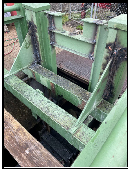
Figure 2: Driscoll Construction began to cut and remove removal of the lifting assemblies on the East side tide gate.
