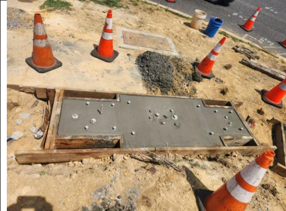
Photo A-1 of 2 Date Taken: June 13, 2024. Description: Foundation Type P-MC, STA 6+22, 57' Right (P.S 11 OF 16 Electrical Plan)
