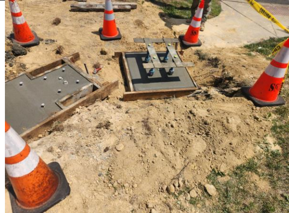
Photo A-2 of 2, Date Taken: June 13, 2024 Description: Foundation Type STF, STA 6+25, 61' Right (P.S 11 OF 16 Electrical Plan)
