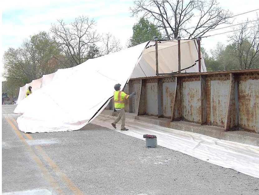
Workers set up the pollution control system prior to sand blasting the girders
