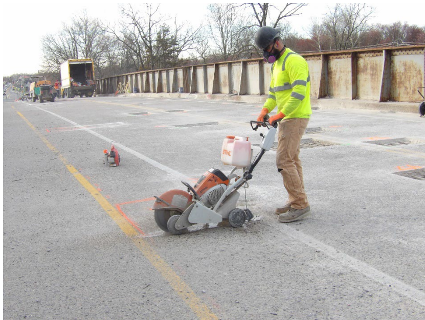
Photo 1 – Workers continued to saw-cut deteriorated marked-out areas from the top of the deck
