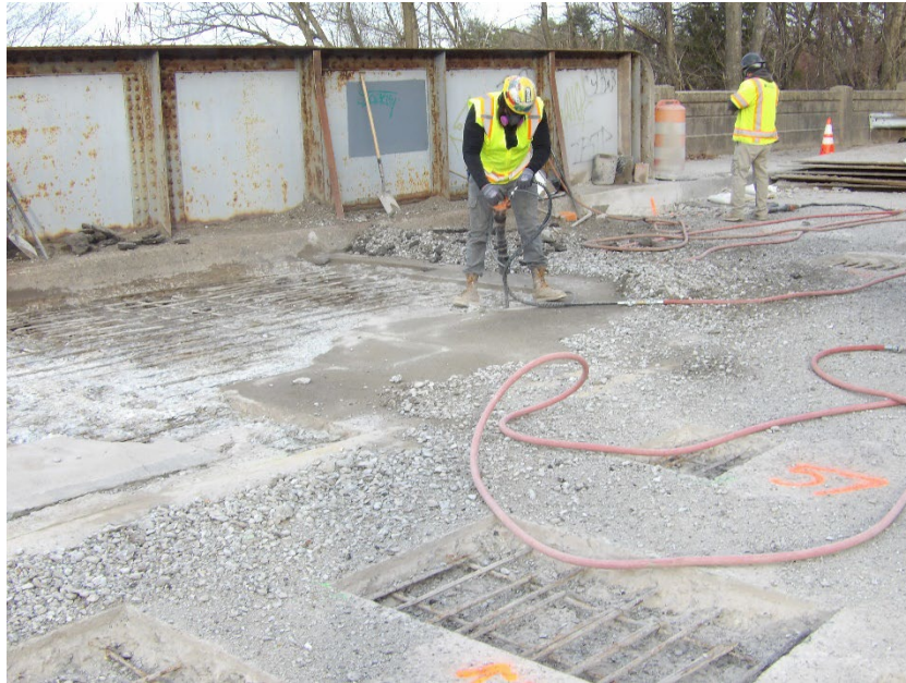
Photo 2 – Workers continued to chip and remove deteriorated concrete from the top of the deck
