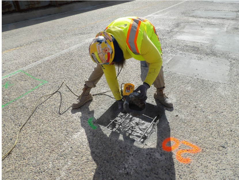
Photo 4 – Workers sprayed areas with a concrete bonding agent prior to pouring new concrete
