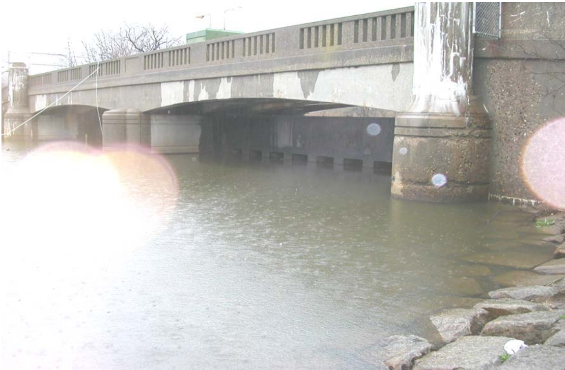
Cooper River Parkway Dam at Kaighn Avenue in Camden City: the tide gates prevent flow upstream during a high tide.
