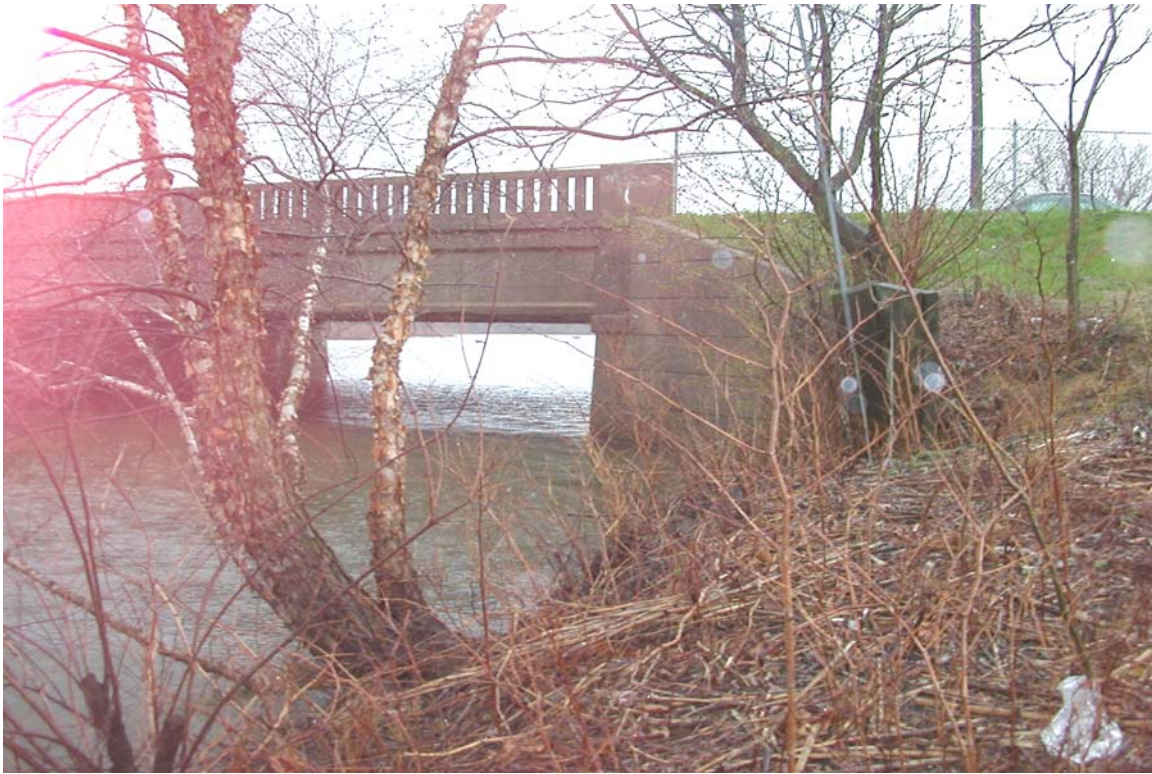
Cooper River Lake at Route 130 bridge, Collingswood. View on the Cooper River Lake from the east side toward west
