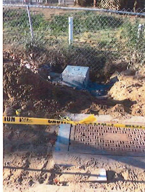
Figure 3: Traffic Signal Foundation
