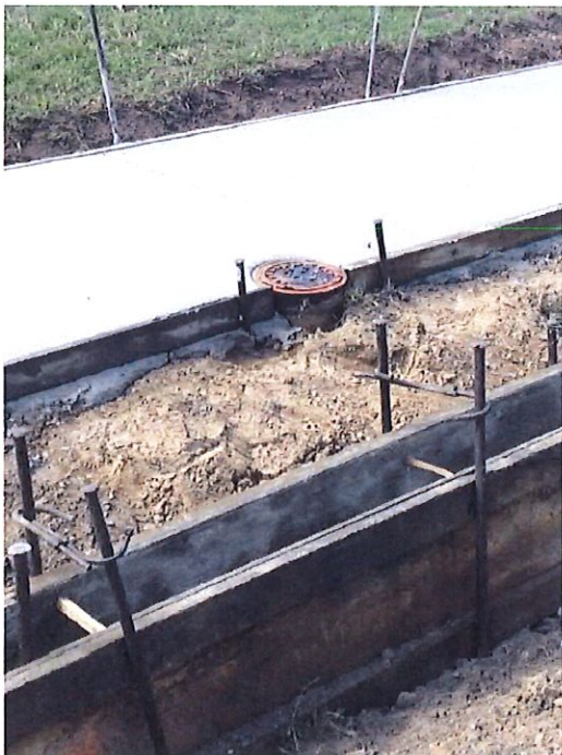
Figure 4: Reset Gas Valve Box
