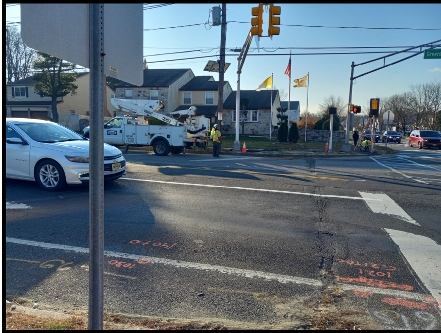
Photograph 9 – Electrical subcontractor activating new traffic signals at the S. Birchwood Park Drive intersection and beginning to remove old hardware.
