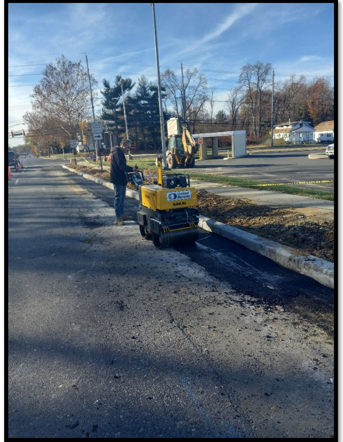
Photograph 4 – Asphalt restorations being completed adjacent to new concrete curb utilizing a small drum roller.
