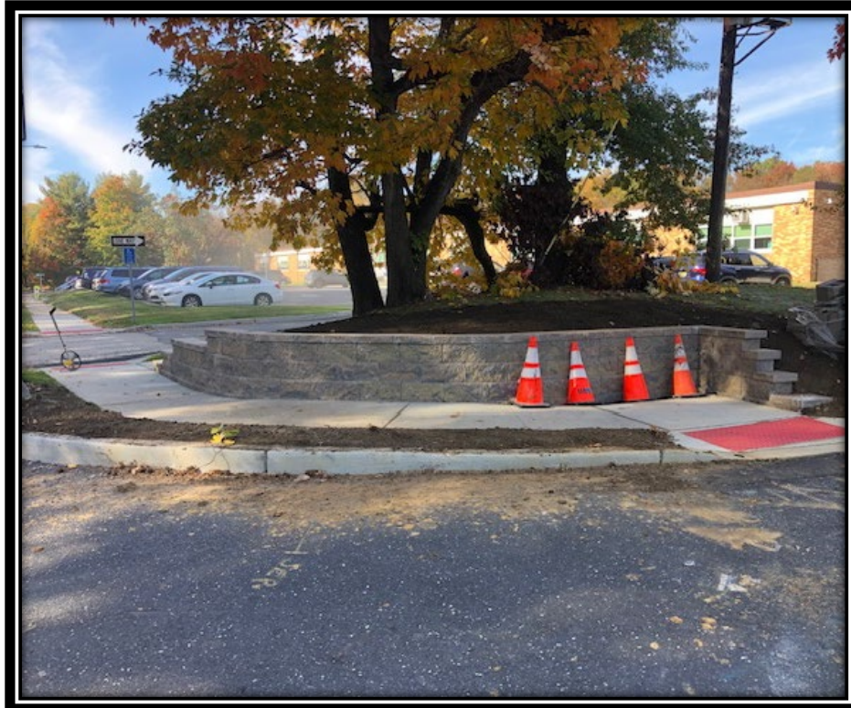
Figure: 3 – Installation of block retaining wall at the intersection with Crofton Commons
