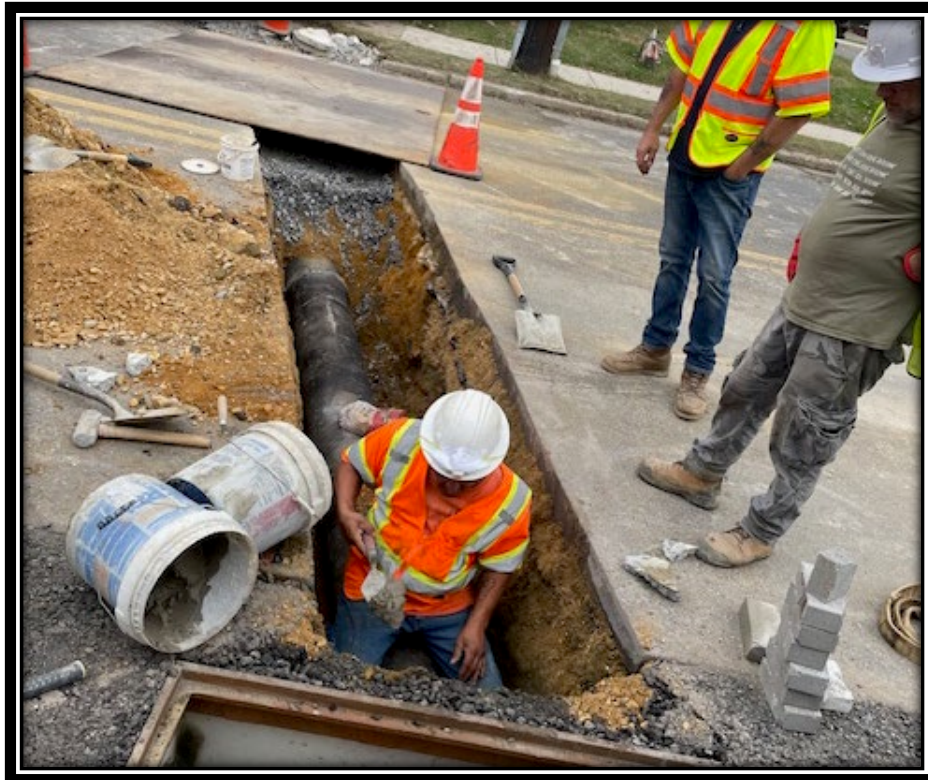
Figure: 2 – Installation of 12” DIP and Type ‘A’ inlet between Oak Avenue and NJSH Rt. 38
