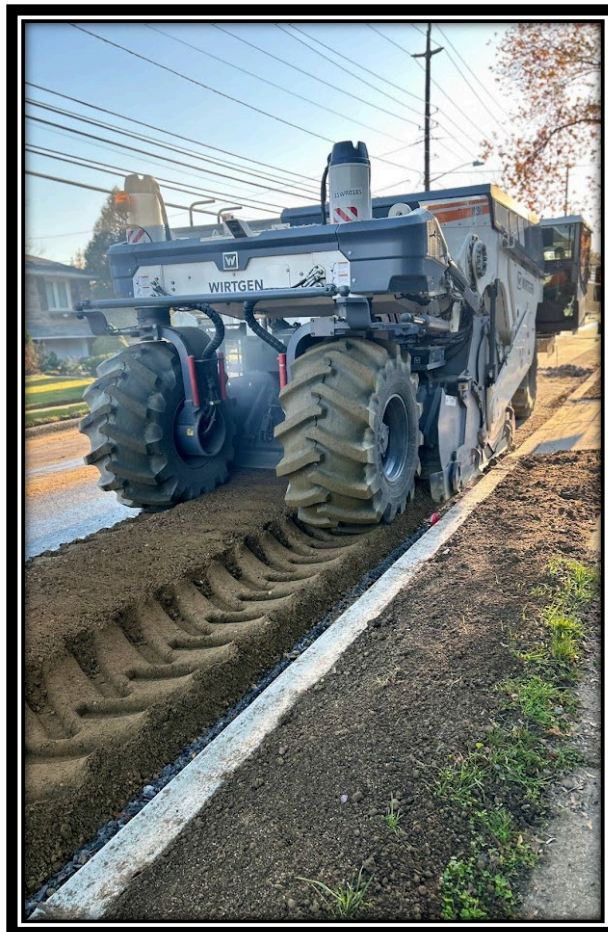
Figure: 1 – Full depth reclamation with cement along the eastbound lane between Columbia Boulevard and Plum Court
