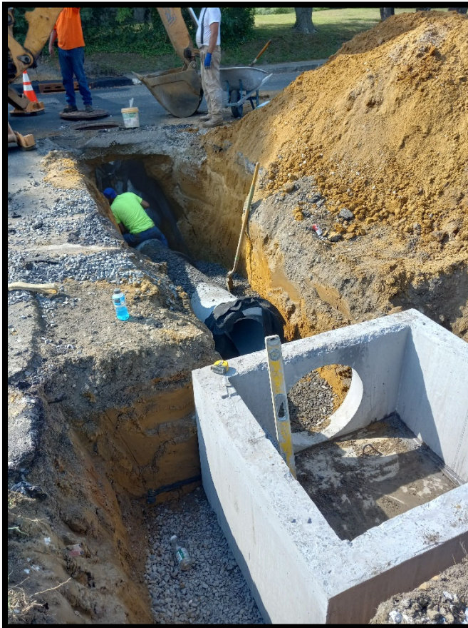
Photograph 1 – Pipe subcontractor installing new “B” inlet and 15” RCP cross drain at Station 147+40L.
