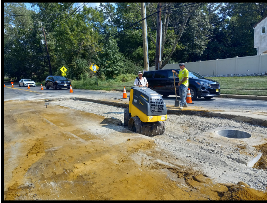
Photograph 5 – Pipe subcontractor performing pavement restoration for trench between Diverter Manhole and Manhole at Station 153+40.
