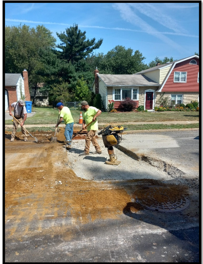
Photograph 2 – Pipe subcontractor performing pavement restoration for trenches at new “B” inlet and 15” RCP cross drain at Station 147+40L.
