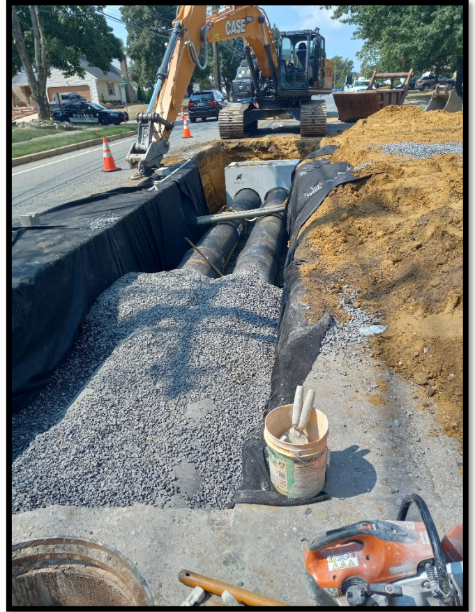
Photograph 4 – Dual 24” Ductile Iron Storm Pipe being installed from Diverter Manhole to Manhole at Station 153+40.
