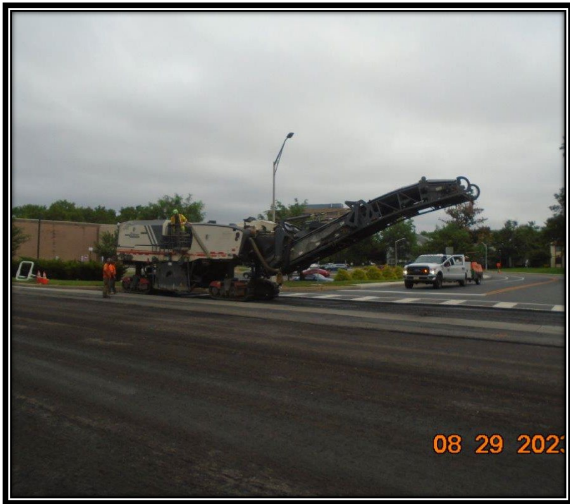
Figure: 1 – HMA milling along the southbound lane between approaching the intersection with Britton Place
