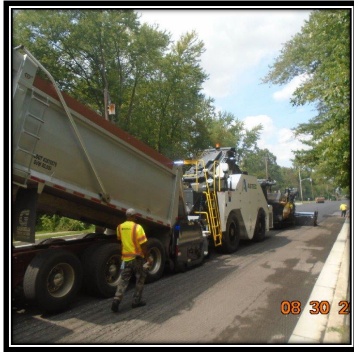
Figure: 2 – Installation of HMA 12.5M64 leveling course along the southbound lane between Britton Place and Cedar Avenue
