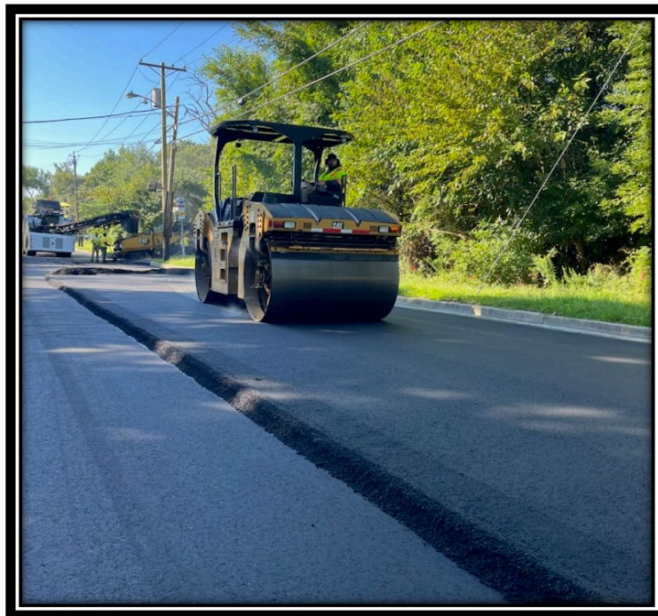
Figure: 3 – Installation of HMA 12.5M64 surface course along the southbound lane between Britton Place and Osage Avenue
