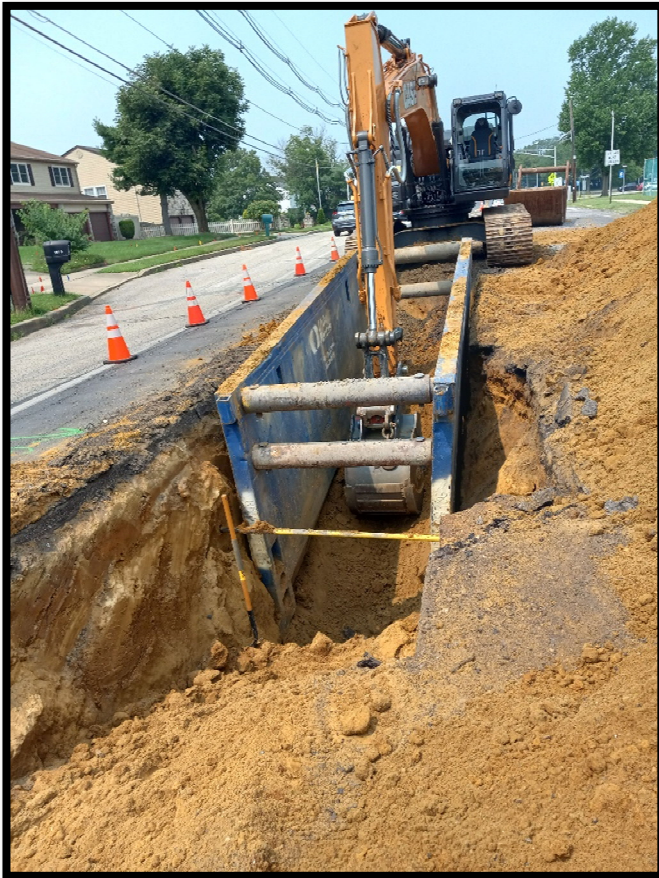
Photograph 1 – The pipe subcontractor is excavating and utilizing a trench box to assist with installation of 15" RCP storm pipe.
