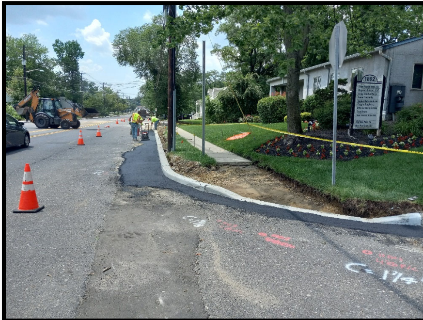
Photograph 6 – Temporary Asphalt restorations being installed adjacent to recently poured concrete vertical curb.
