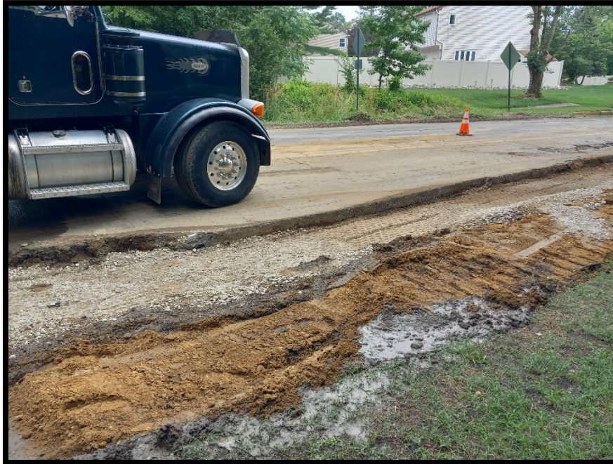
Photograph 3 – Preparing 24" RCP trench at the eastern end of project for Temporary Asphalt Trench Restoration.
