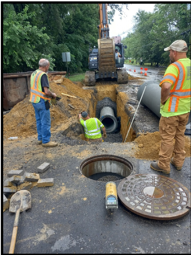
Photograph 1 – The pipe subcontractor continued installing 24” RCP at the eastern end of the project near the County border heading towards the Diverter Manhole.
