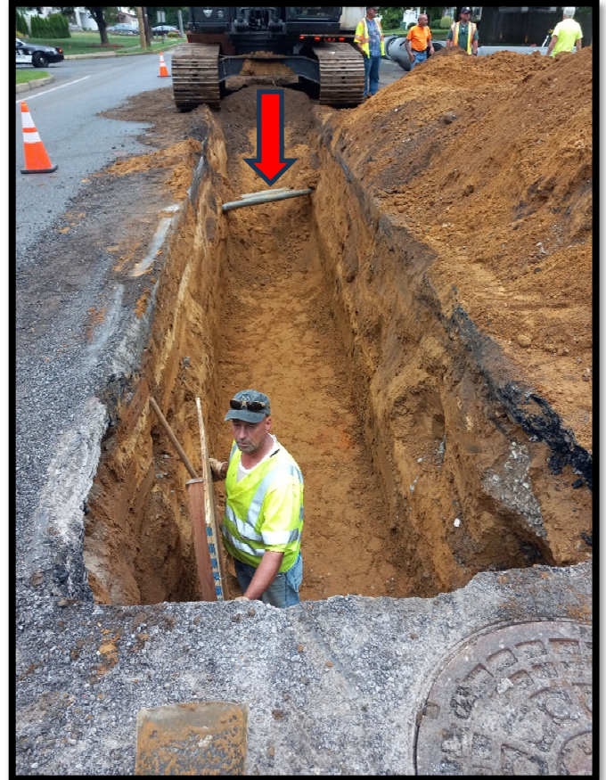
Photograph 6 – Electrical conduits in direct conflict with proposed 30” RCP upstream of the diverter manhole. Trench backfilled and restored without pipe being installed until conflict is resolved.
