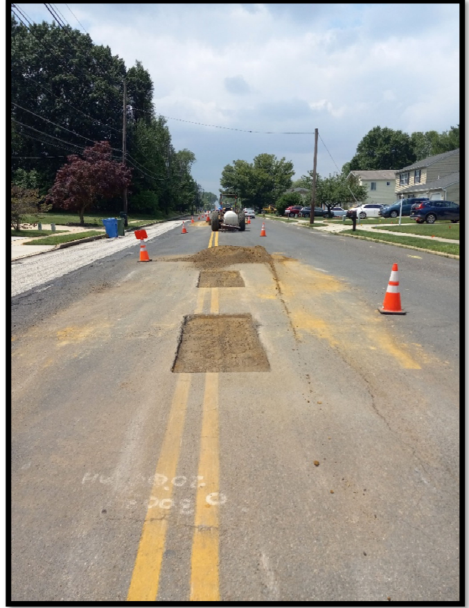
Photograph 8 – Pipe subcontractor restoring roadway at test pit locations after locating underground utilities.
