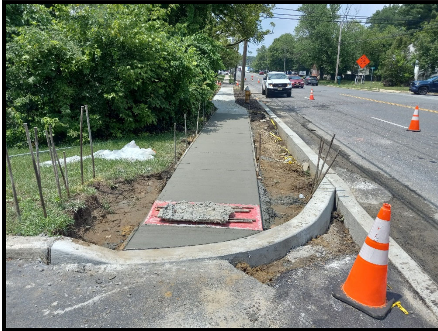
Photograph 9 – Concrete crew continued installing concrete sidewalk and handicapped accessible ramps between Route 70 and Springdale Road.
