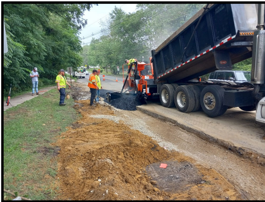
Photograph 4 – Temporary Asphalt Trench Restoration being placed for the 24" RCP at the eastern end of project.
