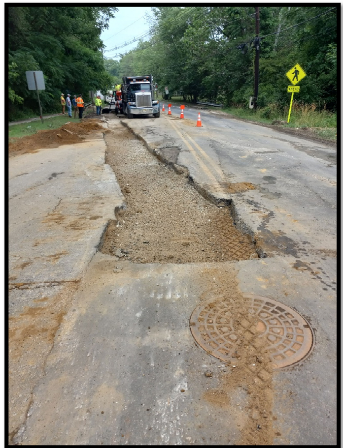
Photograph 2 – Backfilled trench for the 24” RCP at the eastern end of project near the Diverter Manhole.
