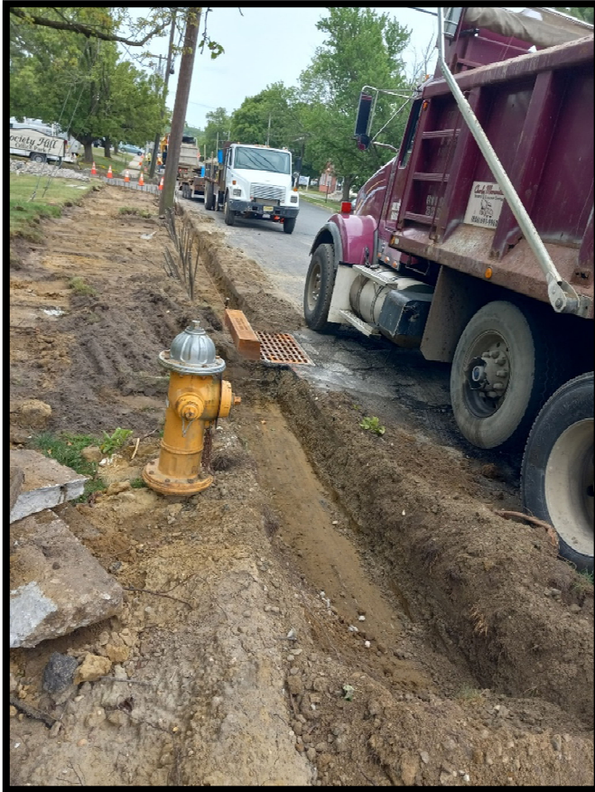
Photograph 3 – The concrete crew began installing concrete curb between Route 70 and Springdale Road.
