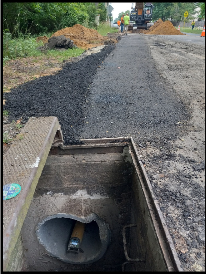
Photograph 3 –24" RCP installed at the eastern end of the project near the County border heading towards the Diverter Manhole. Temporary Asphalt Trench Restorations completed.
