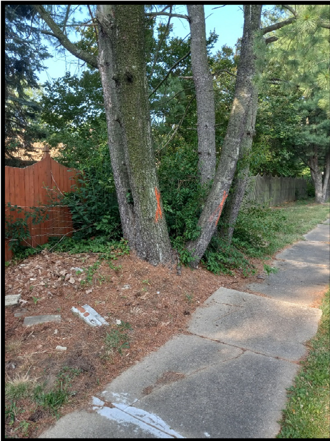
Photograph 1 – The tree subcontractor continued to remove trees in accordance with the Contract Documents.
