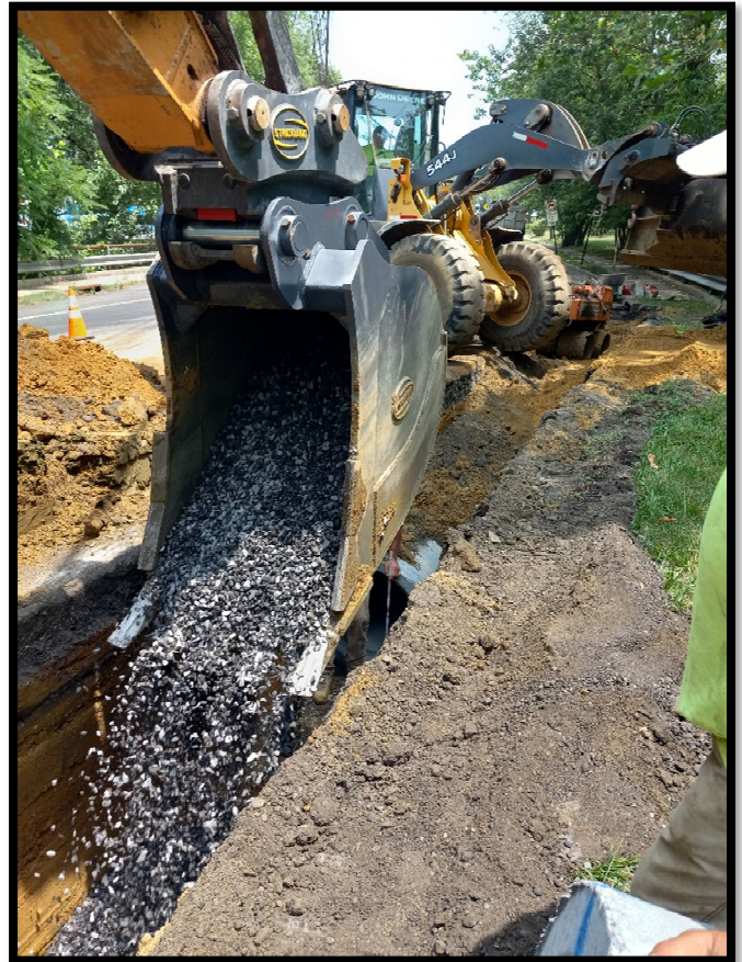
Photograph 2 – The pipe subcontractor began installing 24" RCP at the eastern end of the project near the County border heading towards the Diverter Manhole.
