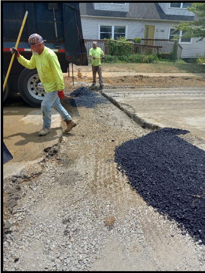
Photograph 3 – Trench restorations for permanent sewer lateral replacements completed at 1883 and 1887 Greentree Road
