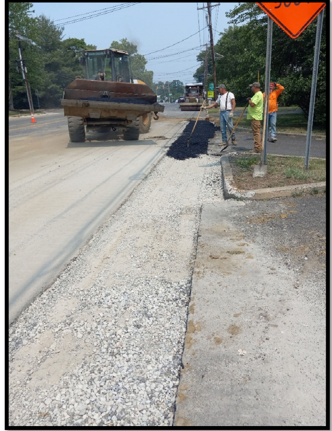
Photograph 6 – Dense Graded Aggregate and Asphalt being installed for Temporary Trench Restoration along the right side of Greentree Road.
