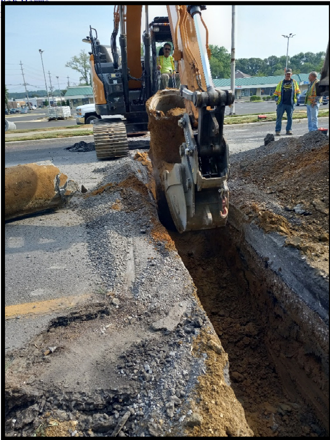
Photograph 7 – Pipe sub-contractor has mobilized to east of Springdale Road to start drainage work.
