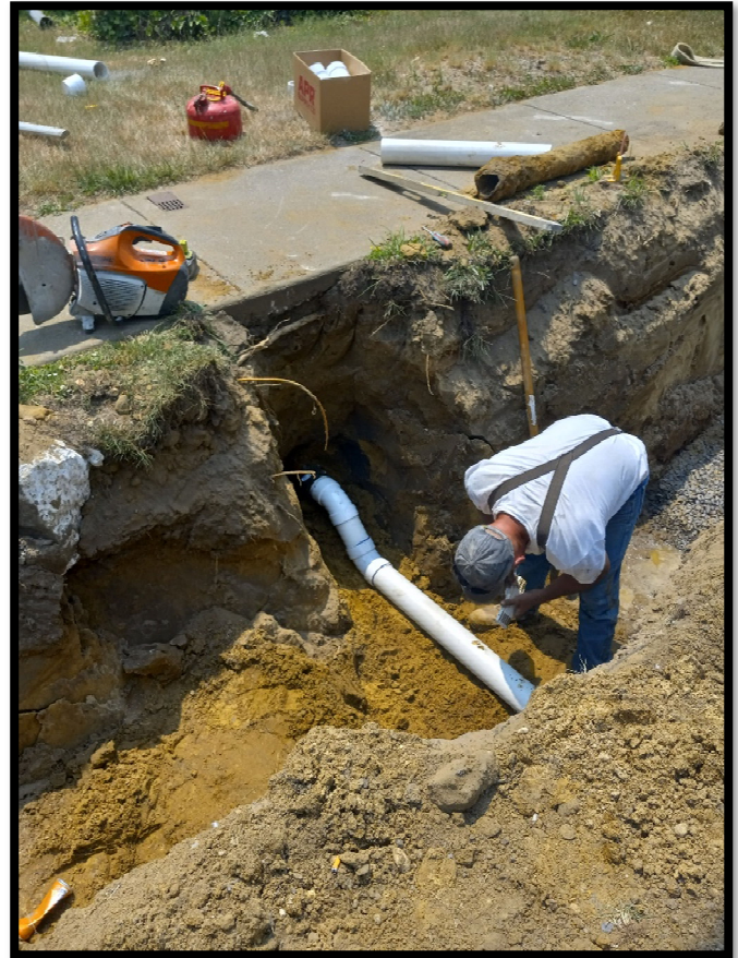
Photograph 4 - Sewer laterals being replaced in order to avoid conflict with 15" RCP at 1883 and 1887 Greentree Road.
