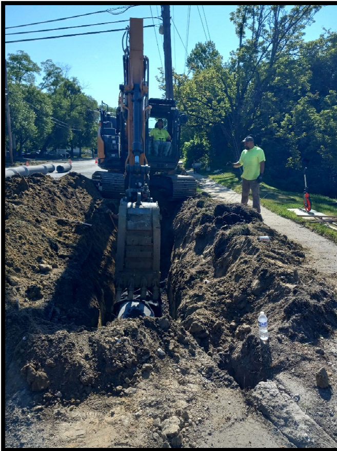
Photograph 1 – The subcontractor performing storm drainage improvements continued installing 15" Class 3 RCP along the right side of Greentree Road.
