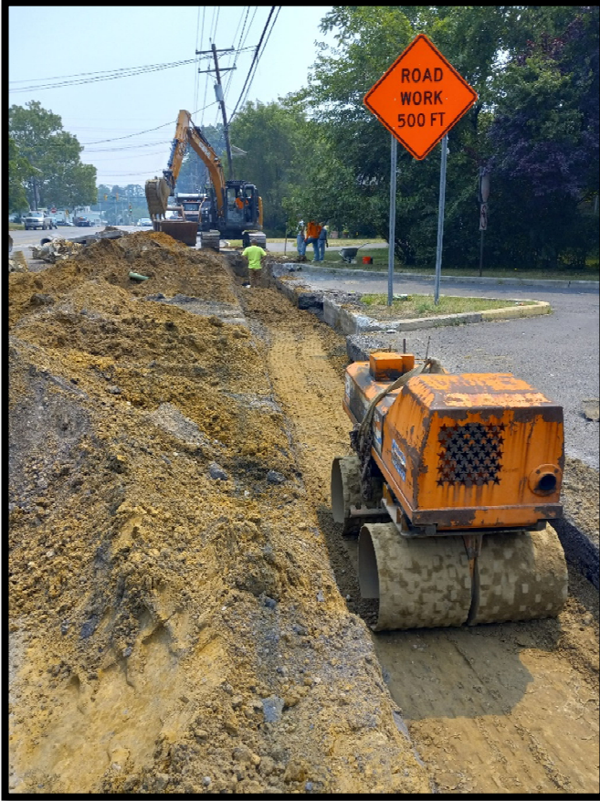
Photograph 5 – Backfilling trench from 15” RCP installation along the right side of Greentree Road.
