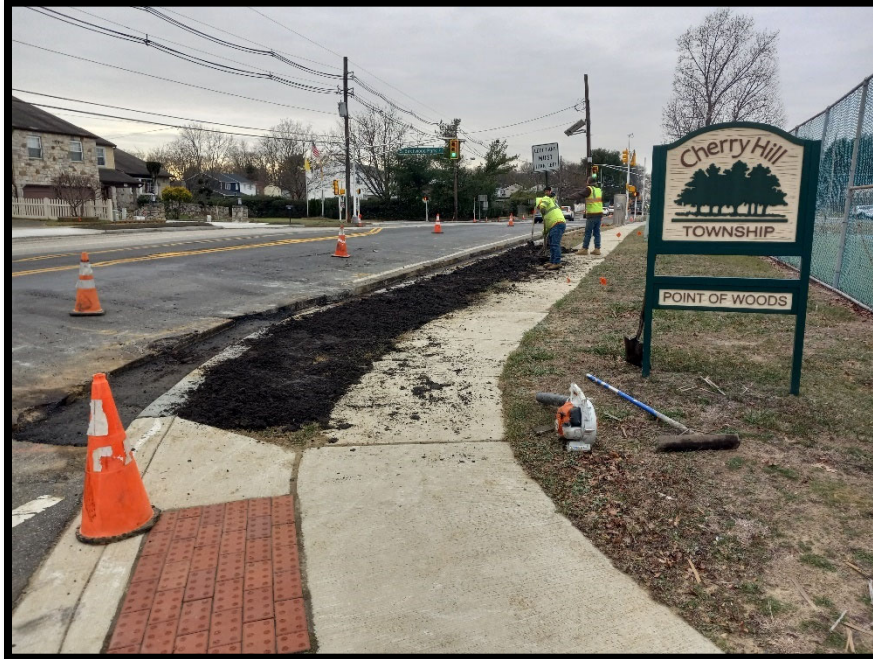
Photograph 5 – Asphalt and topsoil restorations being completed for curb installation in front of Cooper Elementary School tennis courts.
