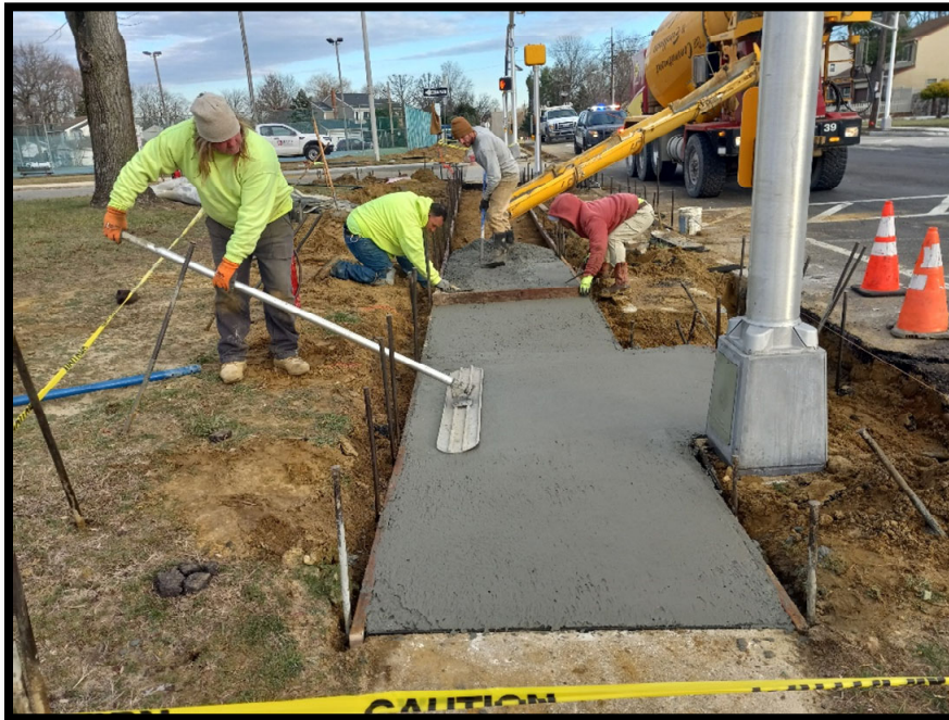
Photograph 4 – Sidewalk and Handicap Accessible Ramps being installed in front of Cooper Elementary School.
