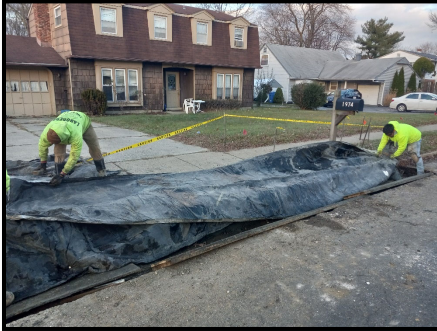
Photograph 3 – Concrete crew installing blankets to protect new driveway apron from overnight freezing temperatures.
