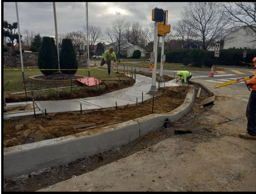
Photograph 5 – Sidewalk and handicap ramps being installed at the S. Birchwood Park Drive intersection.
