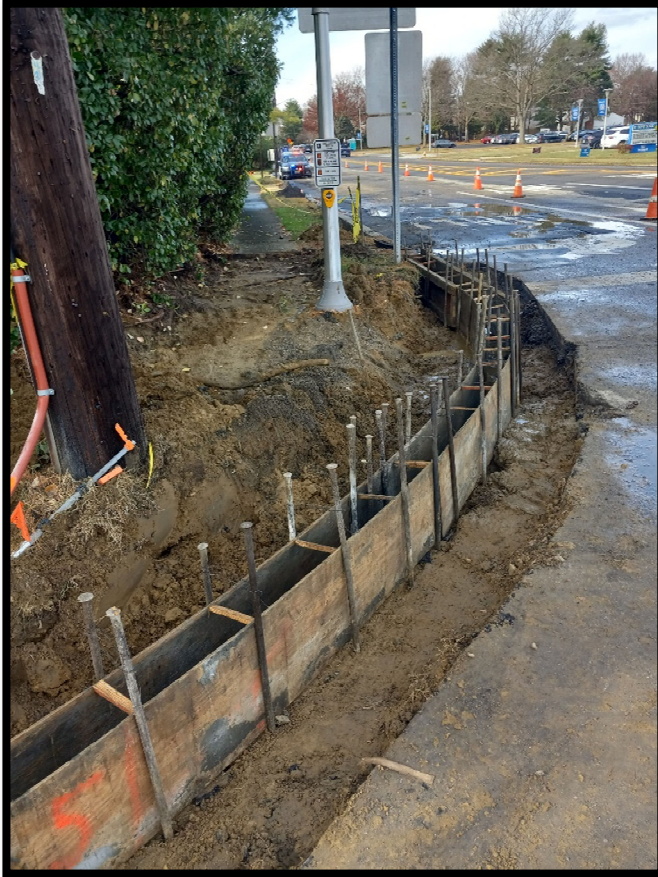
Photograph 1 – Curb forms in place for concrete pour at the S. Birchwood Park Drive intersection.
