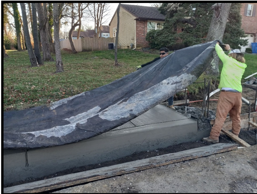
Photograph 6 – Concrete crew installing blankets to protect new sidewalk from overnight freezing temperatures.
