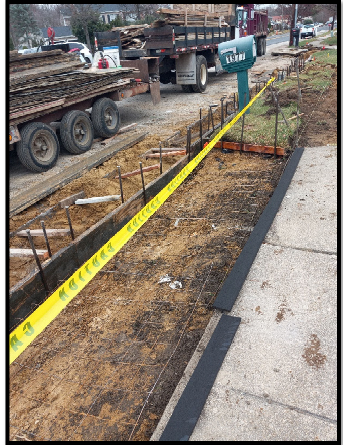
Photograph 4 – Welded wire fabric and expansion joint material being laid out in preparation of concrete pour at 1977 Greentree Road.
