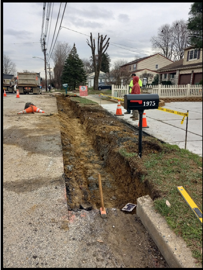
Photograph 3 – Preparing site for concrete curb and driveway apron pour at 1975 and 1977 Greentree Road.
