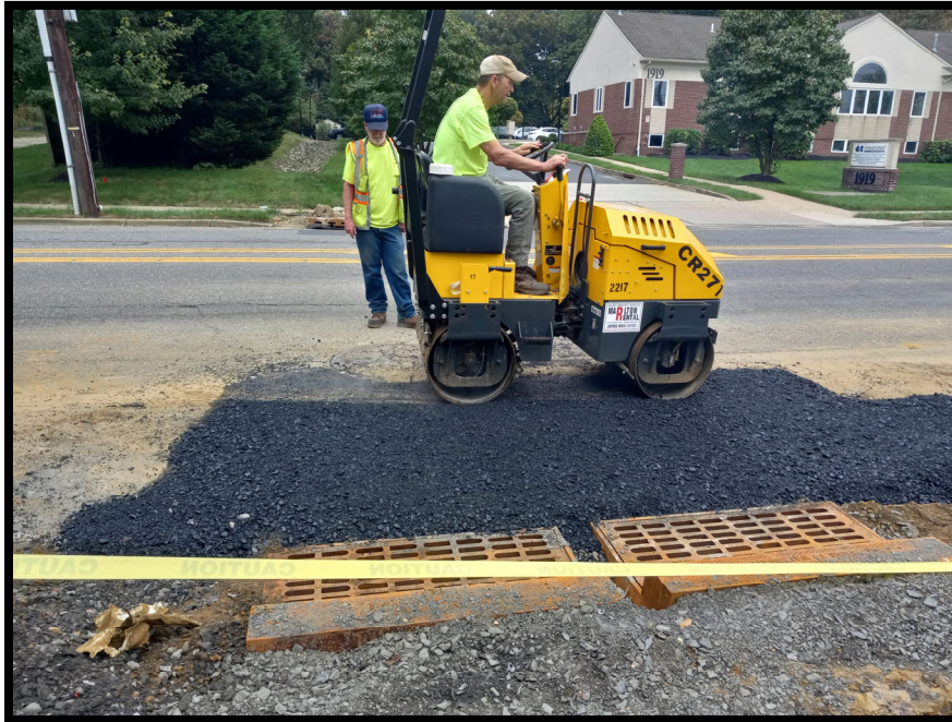
Photograph 5 – Asphalt restorations in front of new Double “B” inlet at Station 122+75L.
