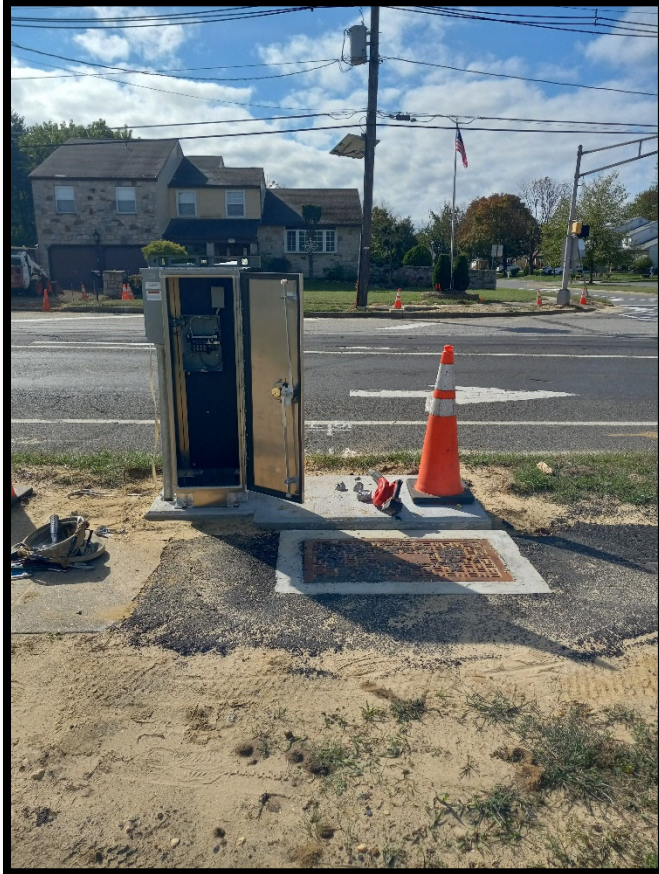
Photograph 3 – Electrical subcontractor setting new control boxes for the traffic signal at South Birchwood Park Drive intersection.
