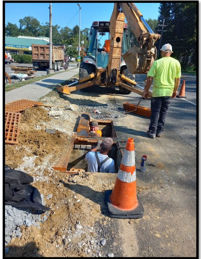
Photograph 2 – Pipe subcontractor setting castings and curb pieces to grade at the new 'B' inlets.
