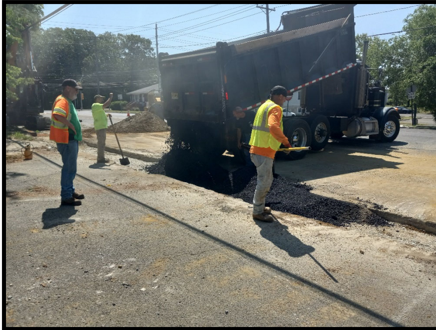
Photograph 5 – Temporary Asphalt Trench Restoration from 15" Class 3 RCP installation along the left side of Greentree Road between Linden Avenue and Princess Avenue.
