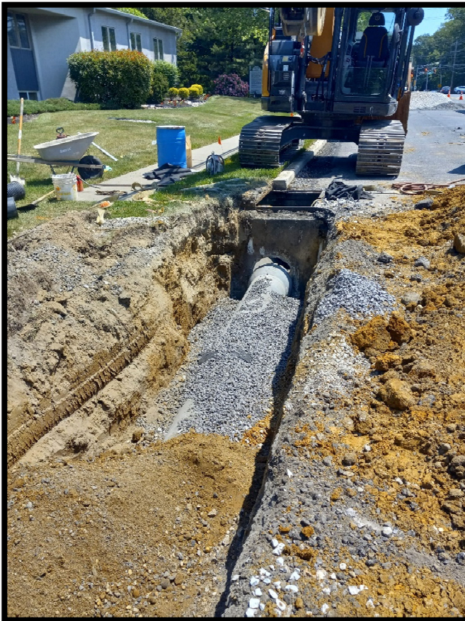
Photograph 1 – The subcontractor performing storm drainage improvements continued installing 15” Class 3 RCP along the left side of Greentree Road between Linden Avenue and Princess Avenue.
