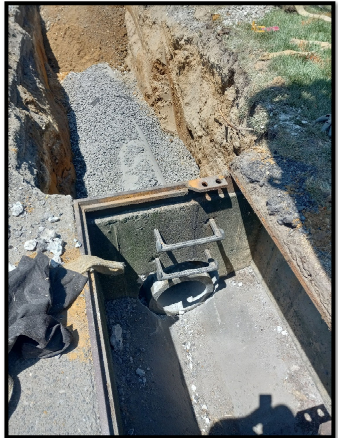
Photograph 2 - 15” Class 3 RCP being tied into an existing inlet near Princess Avenue completing the run from Olney Avenue.
