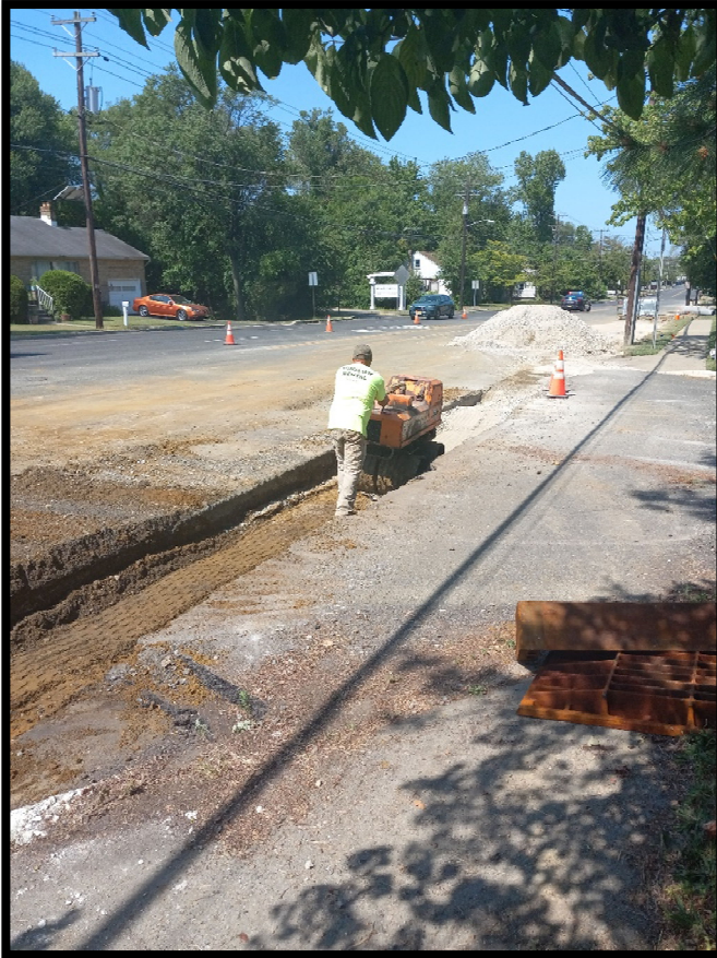
Photograph 3 – Backfilling trench from 15” Class 3 RCP installation along the left side of Greentree Road between Linden Avenue and Princess Avenue.
