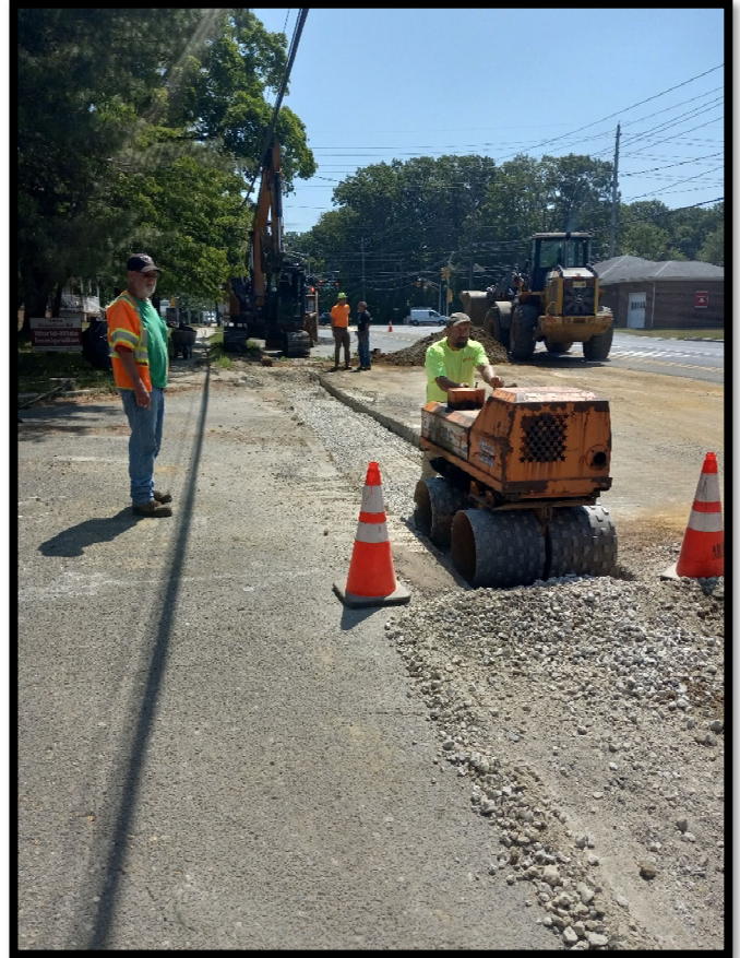
Photograph 4 - Backfilling trench with Dense Graded Aggregate from 15” Class 3 RCP installation along the left side of Greentree Road between Linden Avenue and Princess Avenue.
