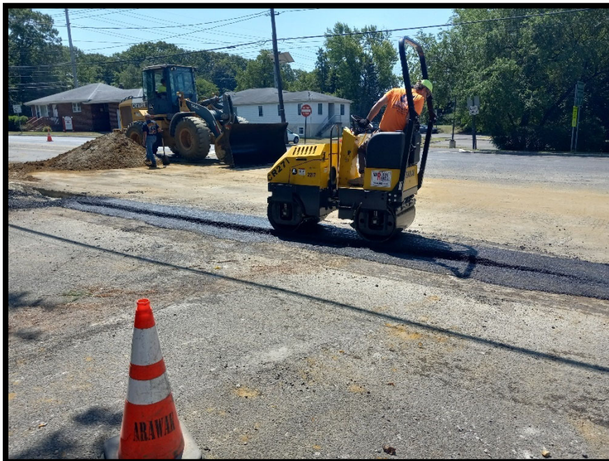
Photograph 6 – Temporary Asphalt Trench Restoration from 15" Class 3 RCP installation along the left side of Greentree Road between Linden Avenue and Princess Avenue.
