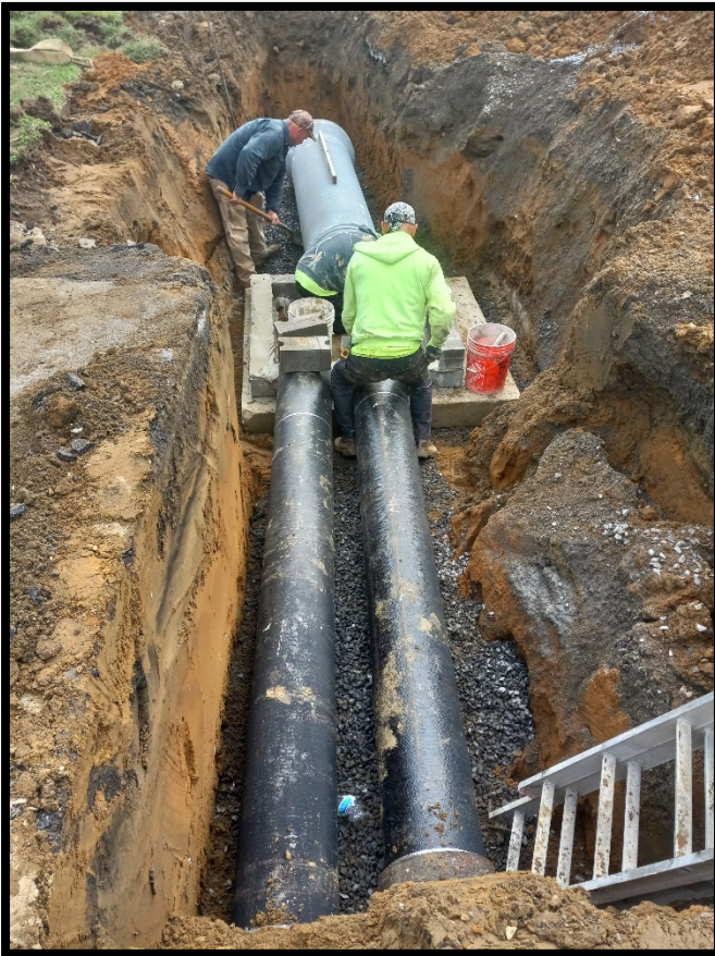
Photograph 1 – Pipe subcontractor installing 'B' inlet at Station 121+80L for transitioning between 18" RCP upstream and dual 12" DIP downstream.
