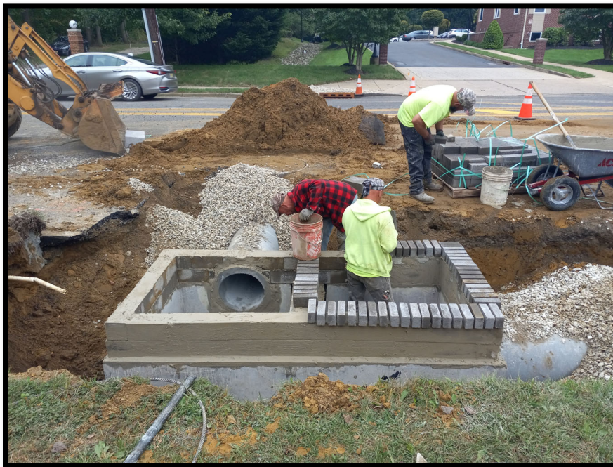
Photograph 6 – Leveling course of block being installed at Double 'B' inlet at Station 122+75L.
