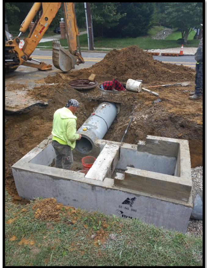
Photograph 4 – 18" RCP storm pipe being installed for existing manhole to new Double 'B' inlet at Station 122+75L.
