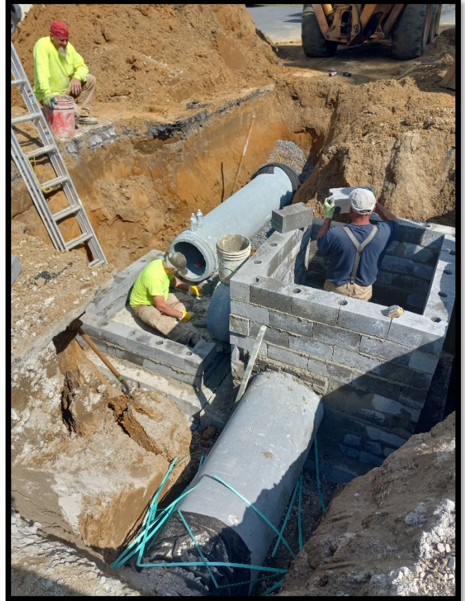
Photograph 4 – Blockwork continues for “B” Inlet at Station 120+75L. Two courses of block installed for adjacent manhole.
