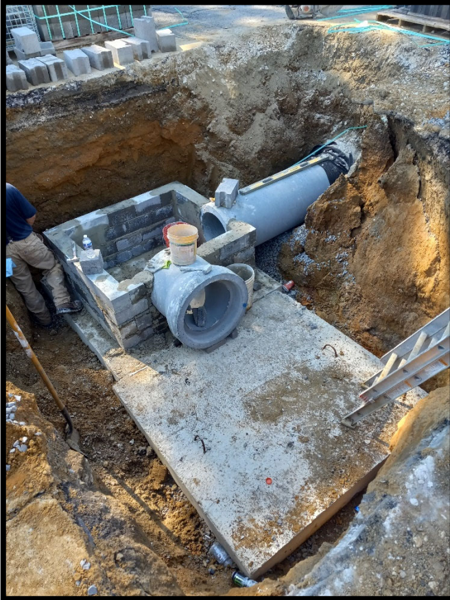
Photograph 3 – Precast slabs in place for “B” inlet and manhole being installed at Station 120+75L. Four courses of block installed for “B” inlet.
