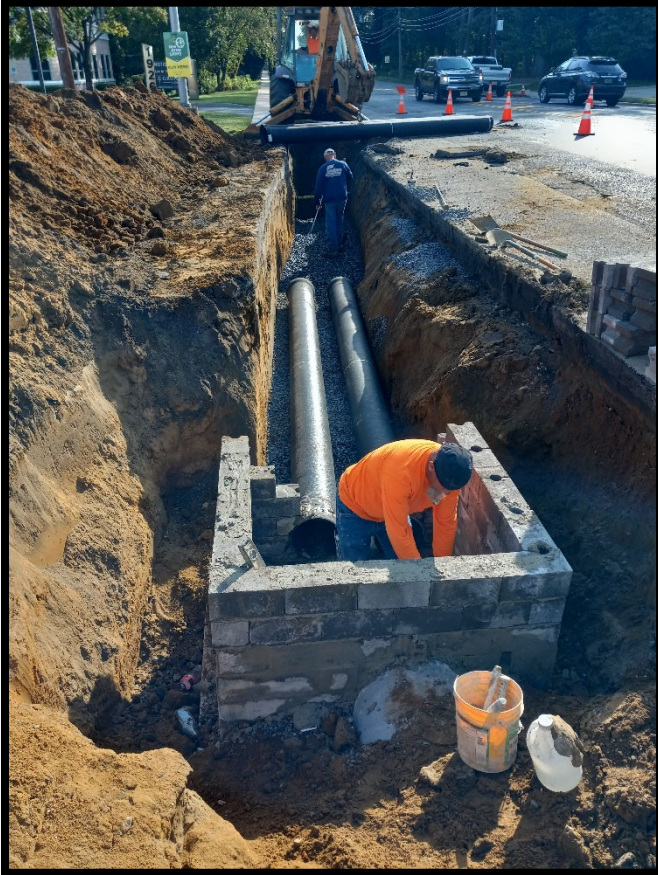
Photograph 7 – 18” RCP downstream and dual 12” DIP storm pipe upstream of the new manhole at Station 121+20L.
