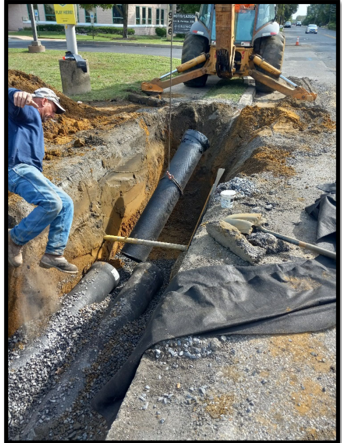
Photograph 8 – Dual 12” DIP storm pipe being installed to go under the 2” gas main servicing the Springdale Plaza Shopping Center.
