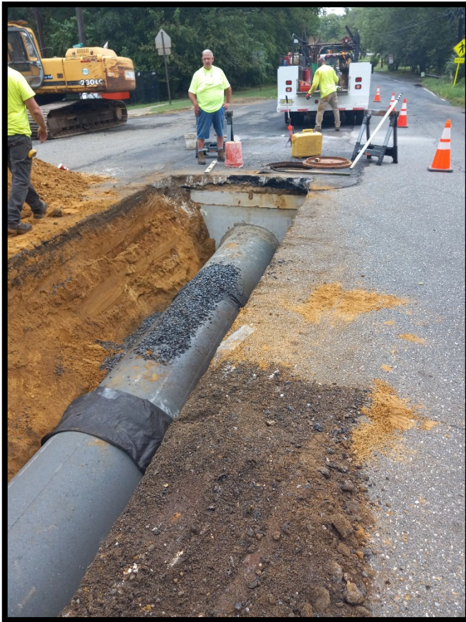
Photograph 1 – Pipe subcontractor installing 30" RCP storm pipe between manholes at Station 153+40 and 147+40L.
