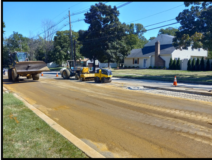
Photograph 3 – Pipe subcontractor completing trench restoration above 30" RCP storm pipe installed between manholes at Station 153+40 and 147+40L.
