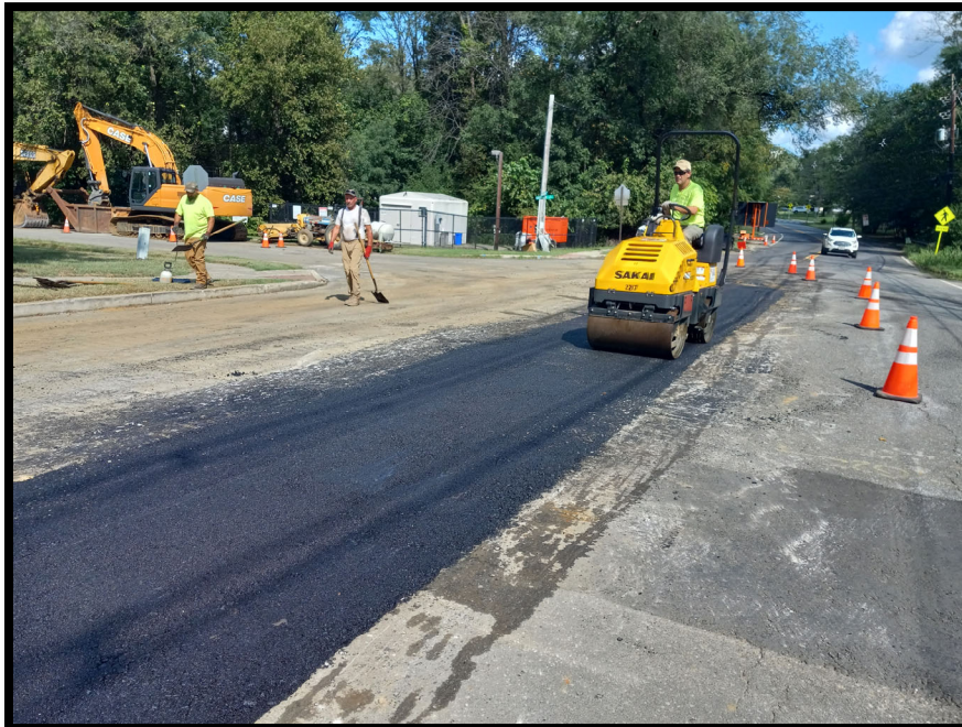
Photograph 4 – Pipe subcontractor completing trench restoration above 30" RCP storm pipe installed between manholes at Station 153+40 and 147+40L.
