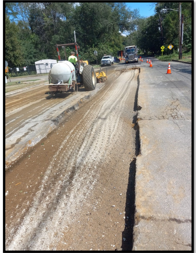
Photograph 2 – Pipe subcontractor completing trench restoration above 30" RCP storm pipe installed between manholes at Station 153+40 and 147+40L.
