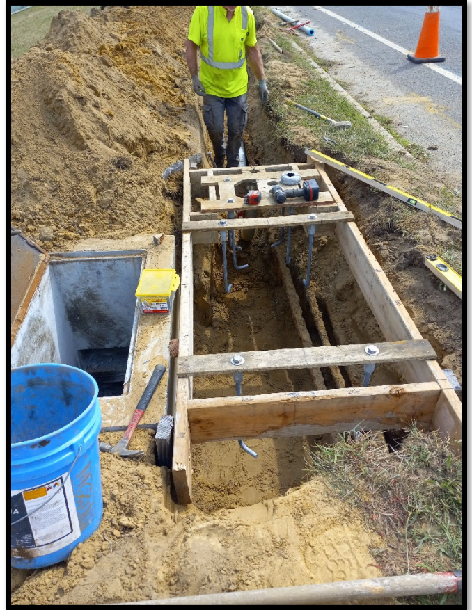
Photograph 4 – Electrical subcontractor installing formwork for concrete foundation pour for traffic signal upgrades at the S. Birchwood Park Drive intersection.
