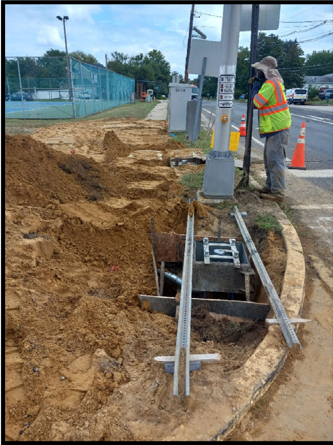
Photograph 8 – Electrical subcontractor installing formwork for concrete foundation pour for traffic signal upgrades at the S. Birchwood Park Drive intersection.
