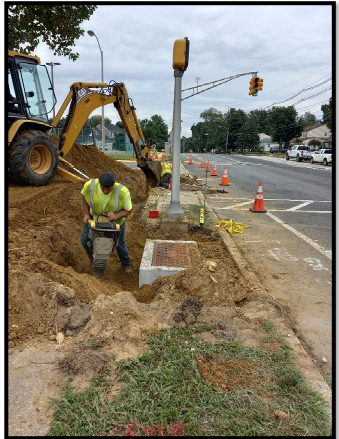
Photograph 7 – Electrical subcontractor backfilling trenches for junction box and rigid metal conduit for traffic signal upgrades at the S. Birchwood Park Drive intersection.
