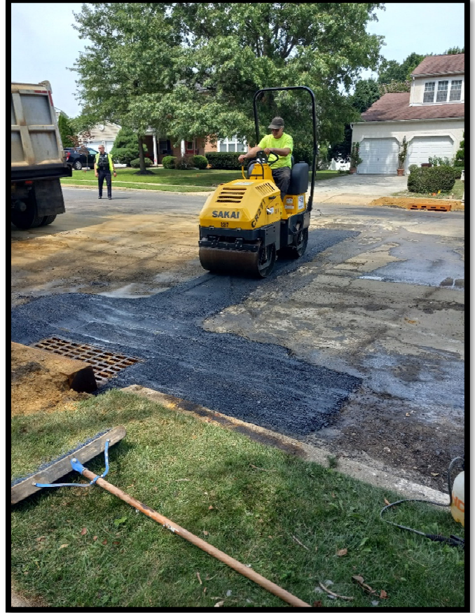
Photograph 5 – Asphalt Trench Restoration for 'B' inlet and corresponding 15" RCP cross drain at Station 144+60R.
