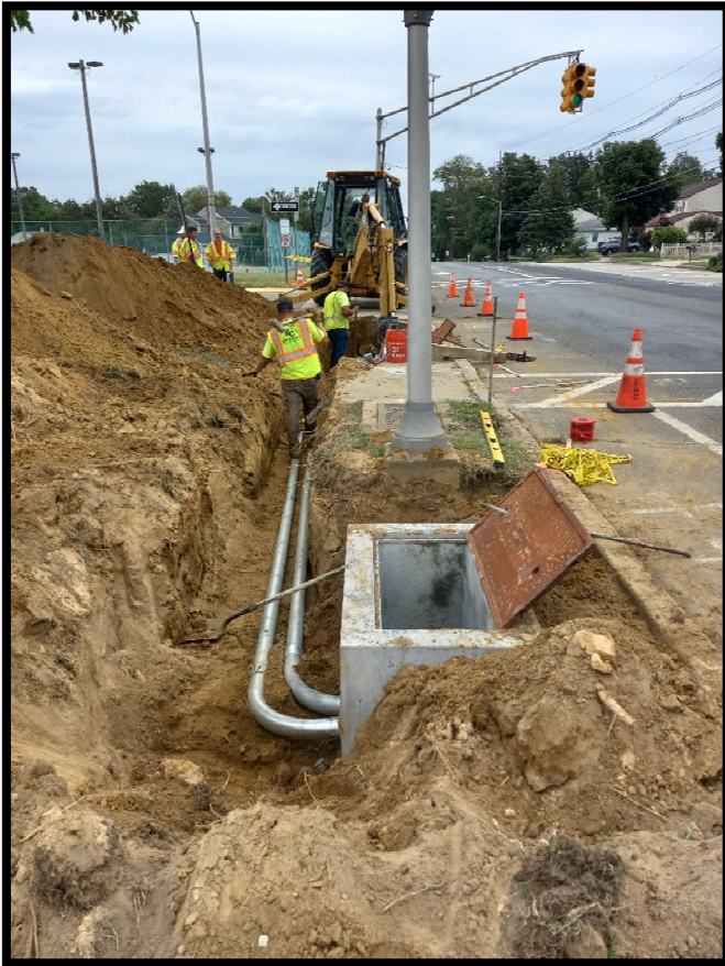
Photograph 6 – Electrical subcontractor installing junction box and rigid metal conduit for traffic signal upgrades at the S. Birchwood Park Drive intersection.
