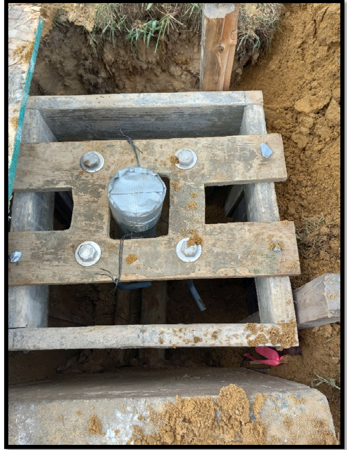
Photograph 9 – Rigid metal conduit, anchor bolts and formwork in place for concrete foundation pour for traffic signal upgrades at the S. Birchwood Park Drive intersection.
