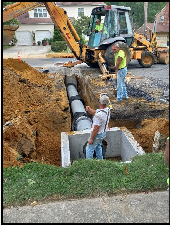
Photograph 4 – Pipe subcontractor installing 'B' inlet and corresponding 15" RCP cross drain at Station 144+60R.
