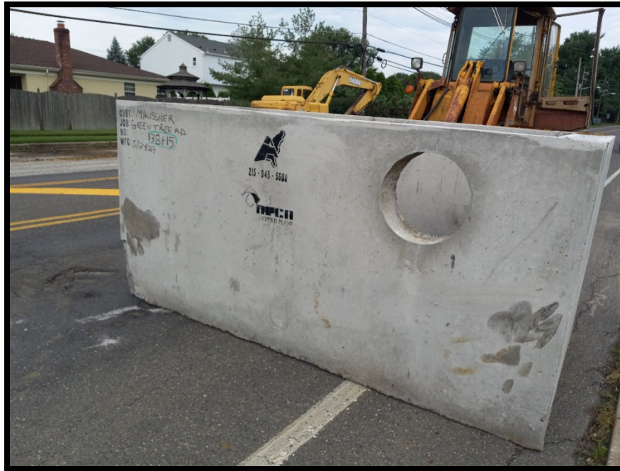
Photograph 1 – Structure for Double “B” Inlet at Station 138+15L delivered to the site.
