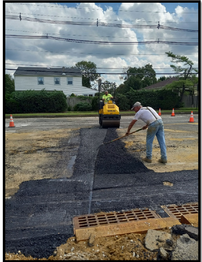
Photograph 5 – Asphalt Trench Restoration for Double “B” Inlet and Cross Drain at Station 138+15L in front of Cooper Elementary School.
