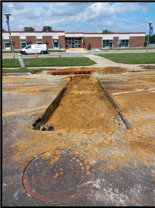
Photograph 4 – Preparing subgrade for Trench Restoration for Double “B” Inlet and Cross Drain at Station 138+15L in front of Cooper Elementary School.
