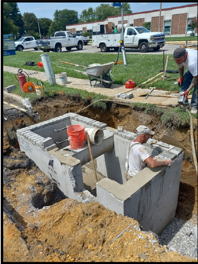
Photograph 2 – Structure for Double “B” Inlet at Station 138+15L installed in front of Cooper Elementary School.
