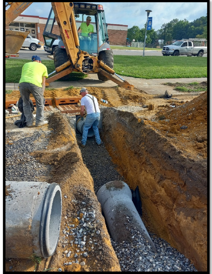
Photograph 3 – 15” RCP storm pipe cross drain being installed from Double “B” Inlet at Station 138+15L to the manhole at the center of Greentree Road in front of Cooper Elementary School.
