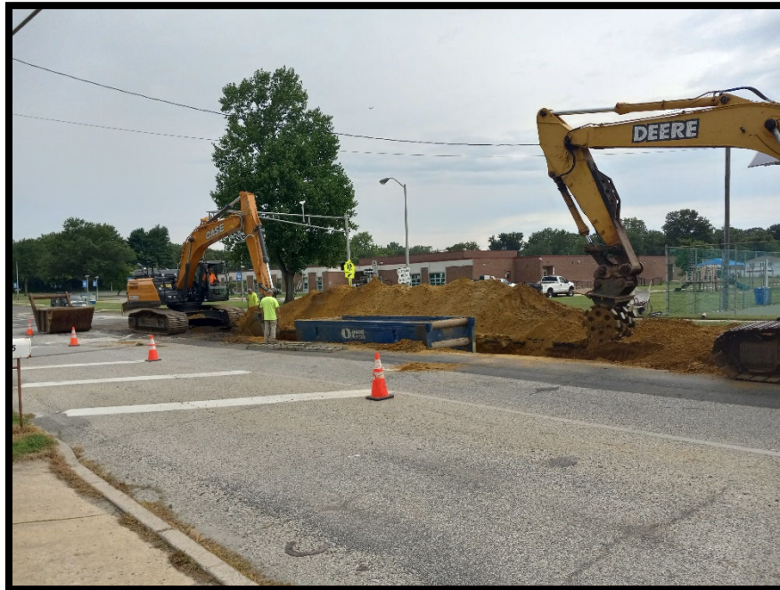
Photograph 1 – The pipe subcontractor is excavating and utilizing a trench box to assist with installation of 15" RCP storm pipe near Cooper Elementary School.
