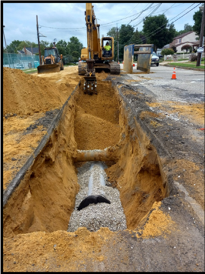
Photograph 2 – The pipe subcontractor is installing 15” RCP storm pipe near Cooper Elementary School.
