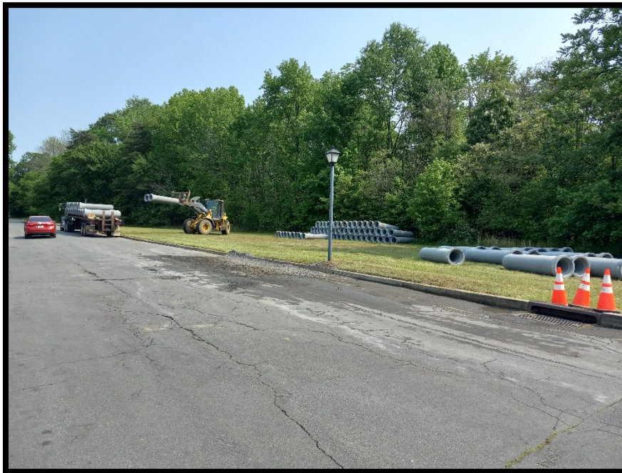
Photograph 1 – Reinforced Concrete Pipe for new drainage system being delivered to lay down yard adjacent to North Green Acre Drive.
