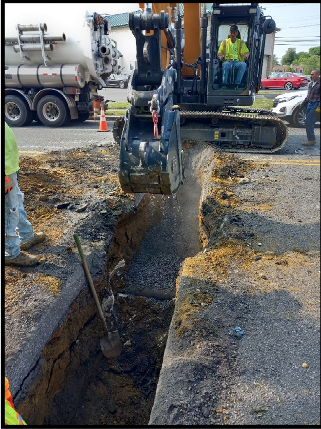
Photograph 4 – Trench excavation for 12” Cement Lined Ductile Iron Pipe for cross-drain from the inlet at Station 103+40L.
