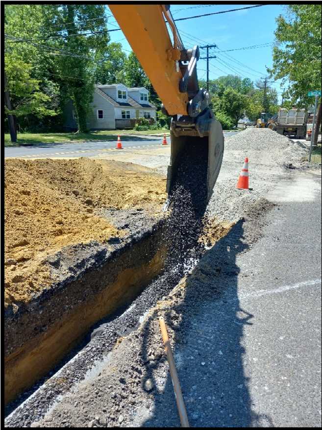
Photograph 10 – Backfilling 15” Class 3 Reinforced Concrete Pipe along the left side of Greentree Road heading east from the inlet at Station 108+60L.
