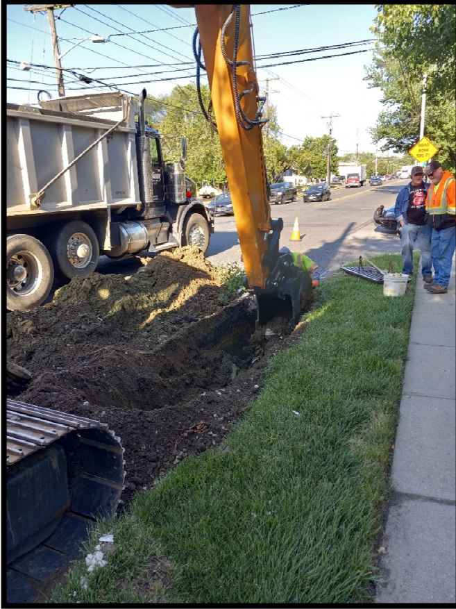
Photograph 8 – Excavating for 15” Class 3 Reinforced Concrete Pipe heading east along the left side of Greentree Road from the inlet at Station 108+60L.
