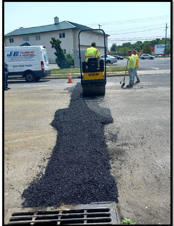
Photograph 7 – Temporary Asphalt Trench Restoration for 12” Cement Lined Ductile Iron Pipe installed for cross-drain from the inlet at Station 103+40L.
