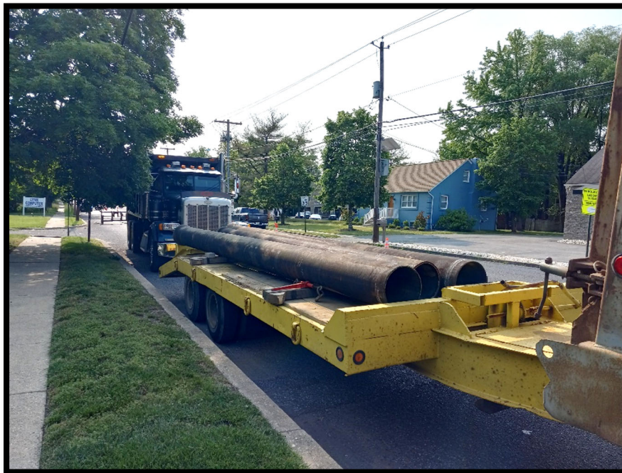
Photograph 3 – Delivery of 12" Cement Lined Ductile Iron Pipe for cross-drain from the inlet at Station 103+40L.
