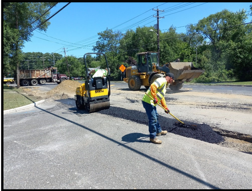
Photograph 14 – Temporary Asphalt Trench Restoration for 15" Class 3 RCP being installed along the left side of Greentree Road heading east from the inlet at Station 108+60L.
