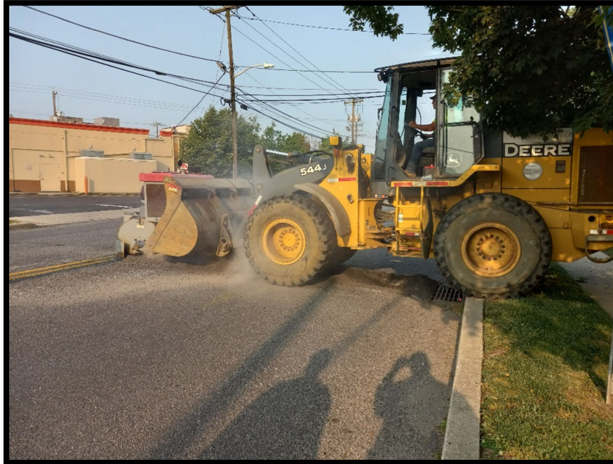
Photograph 2 – Milling trench for installation of 12" Cement Lined Ductile Iron Pipe cross-drain from the inlet at Station 103+40L.
