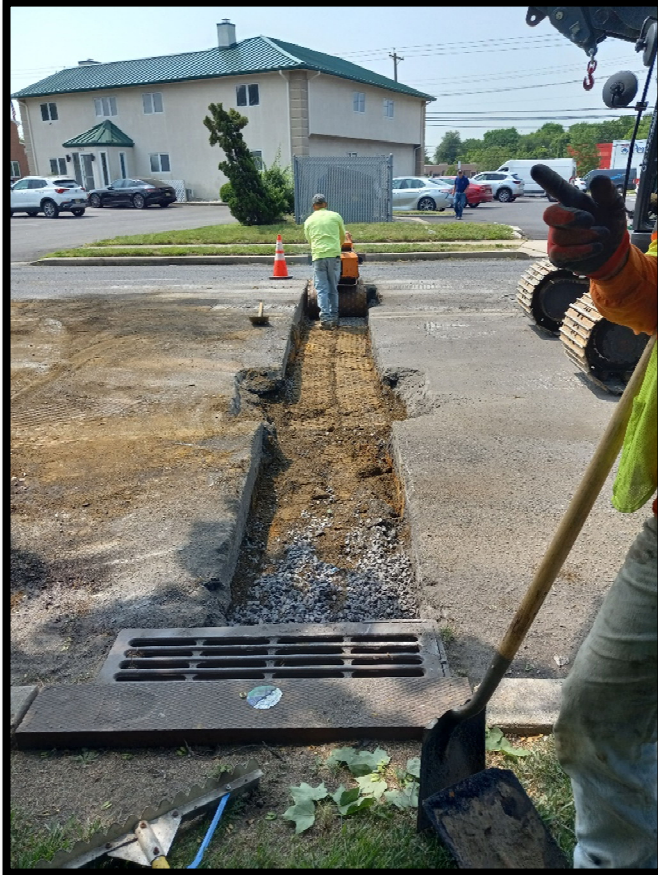
Photograph 6 – Backfilling of trench for 12” Cement Lined Ductile Iron Pipe for cross-drain from the inlet at Station 103+40L.
