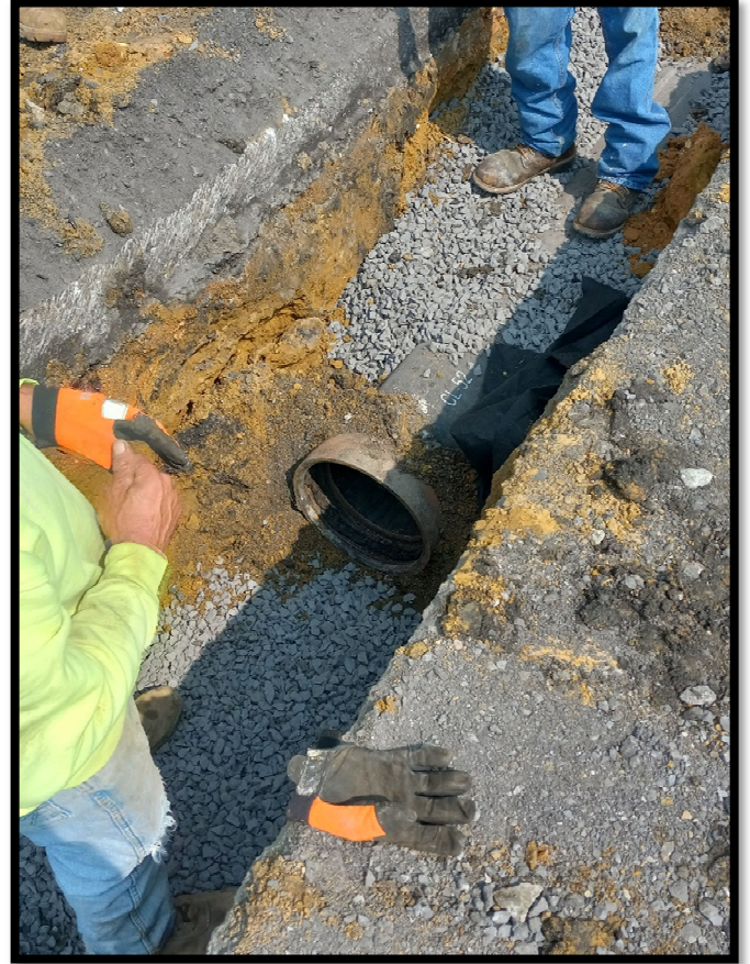
Photograph 5 - 12” Cement Lined Ductile Iron Pipe installed for cross-drain from the inlet at Station 103+40L.
