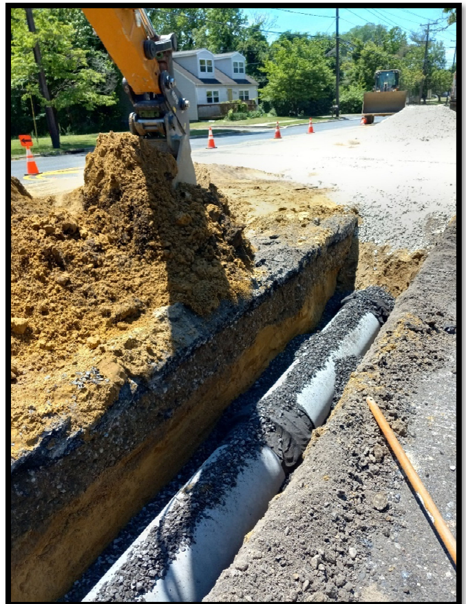
Photograph 11 – Backfilling 15” Class 3 Reinforced Concrete Pipe along the left side of Greentree Road heading east from the inlet at Station 108+60L.
