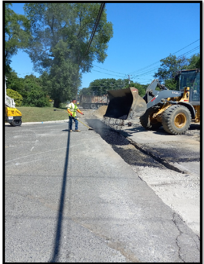
Photograph 13 – Temporary Asphalt Trench Restoration for 15” Class 3 RCP being installed along the left side of Greentree Road heading east from the inlet at Station 108+60L.
