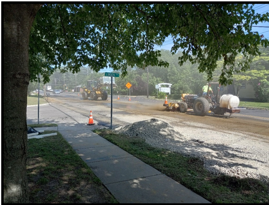
Photograph 15 – Cleaning of dirt and debris from the roadway prior to the weekend
