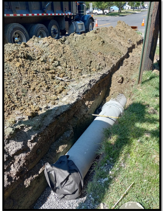
Photograph 9 – 15” Class 3 RCP being installed along the left side of Greentree Road heading east from the inlet at Station 108+60L.
