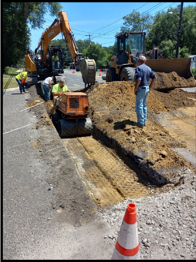
Photograph 12 – Backfilling 15” Class 3 Reinforced Concrete Pipe along the left side of Greentree Road heading east from the inlet at Station 108+60L.
