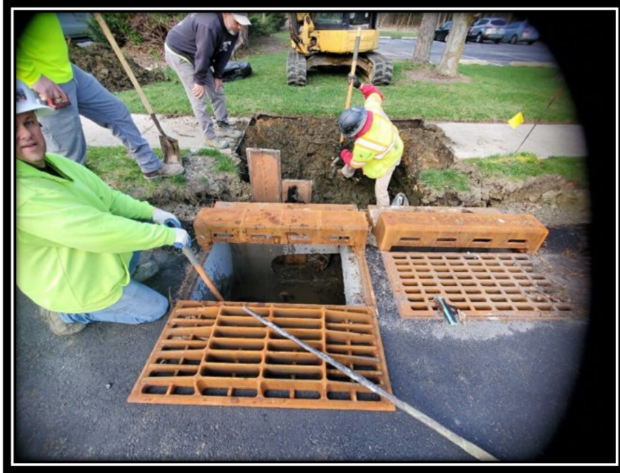
Figure: 2 – Installation of Type Double B Inlet along the southbound lane between Britton Place and Somerdale Road
