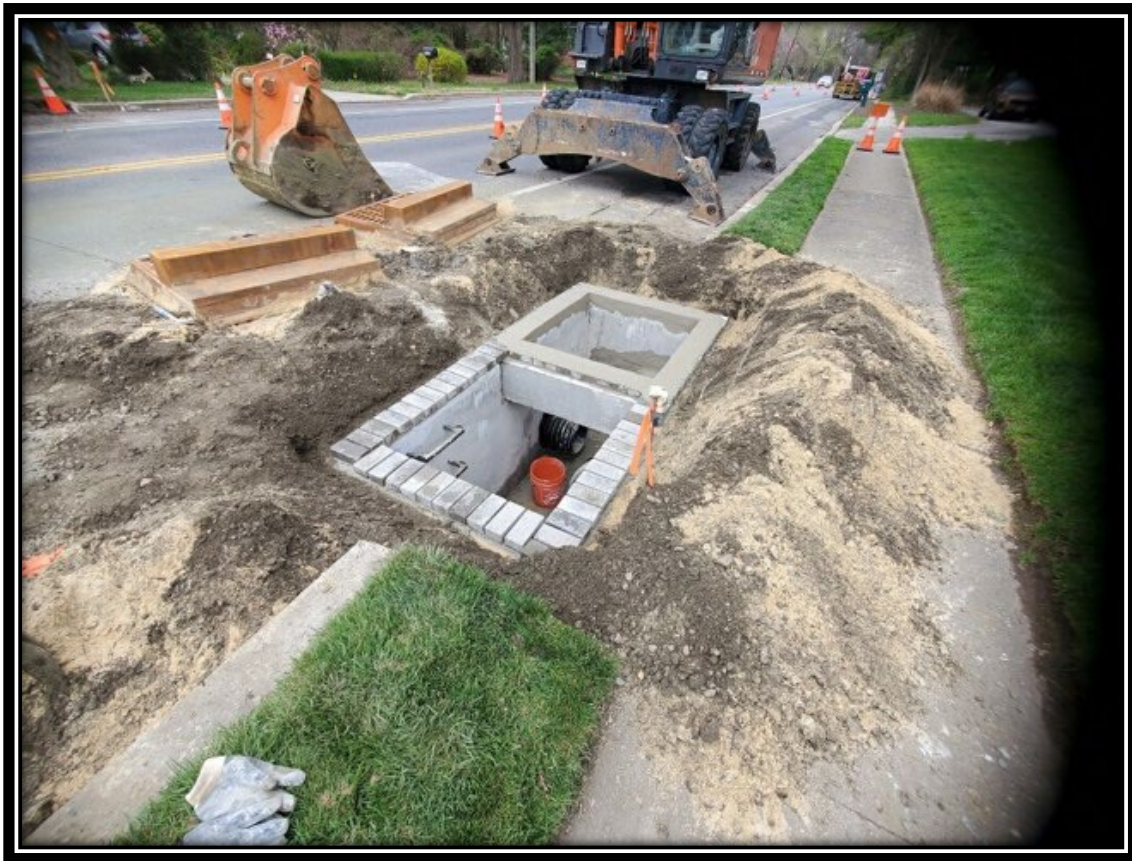
Figure: 1 – Installation of Type Double B Inlet along the northbound lane adjacent to the intersection with Cedar Avenue
