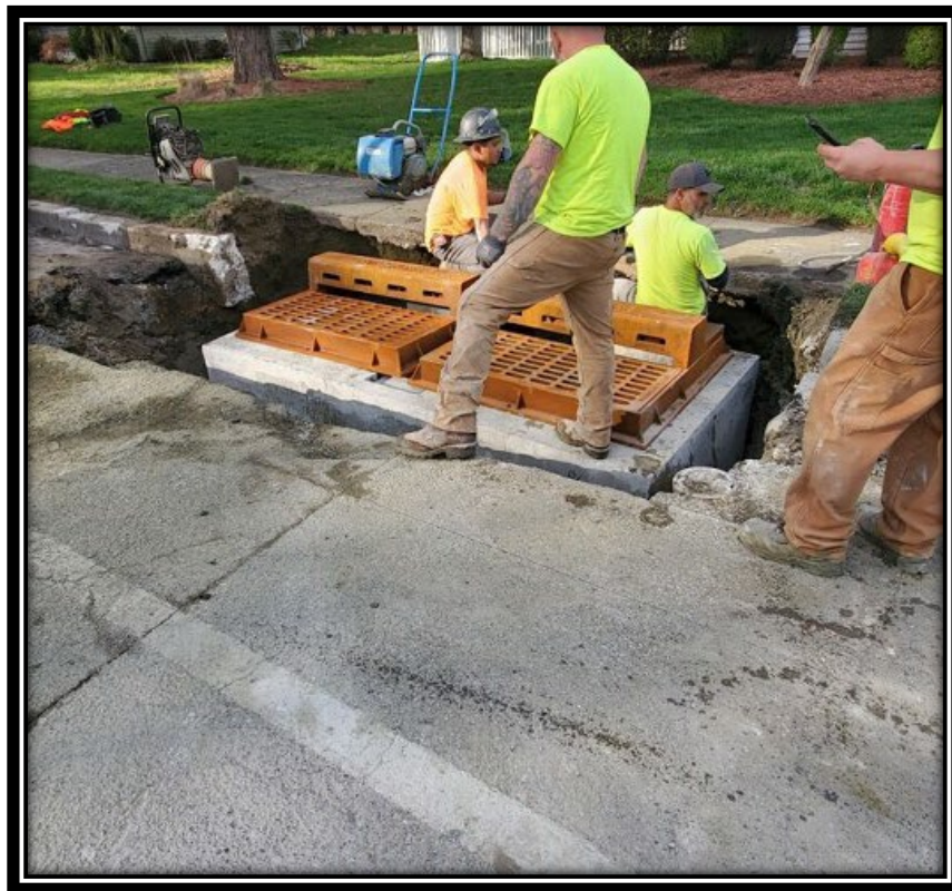
Figure: 3 – Installation of Type Double B Inlet along the northbound lane adjacent to the intersection with Cedar Avenue
