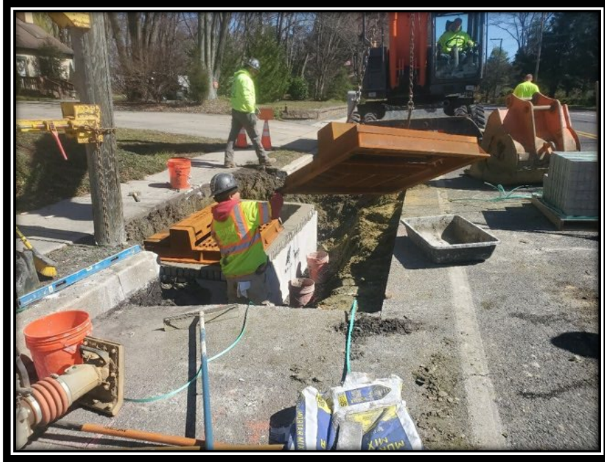
Figure: 2 – Installation of Type Double B Inlet along the northbound lane between Britton Place and Cedar Avenue
