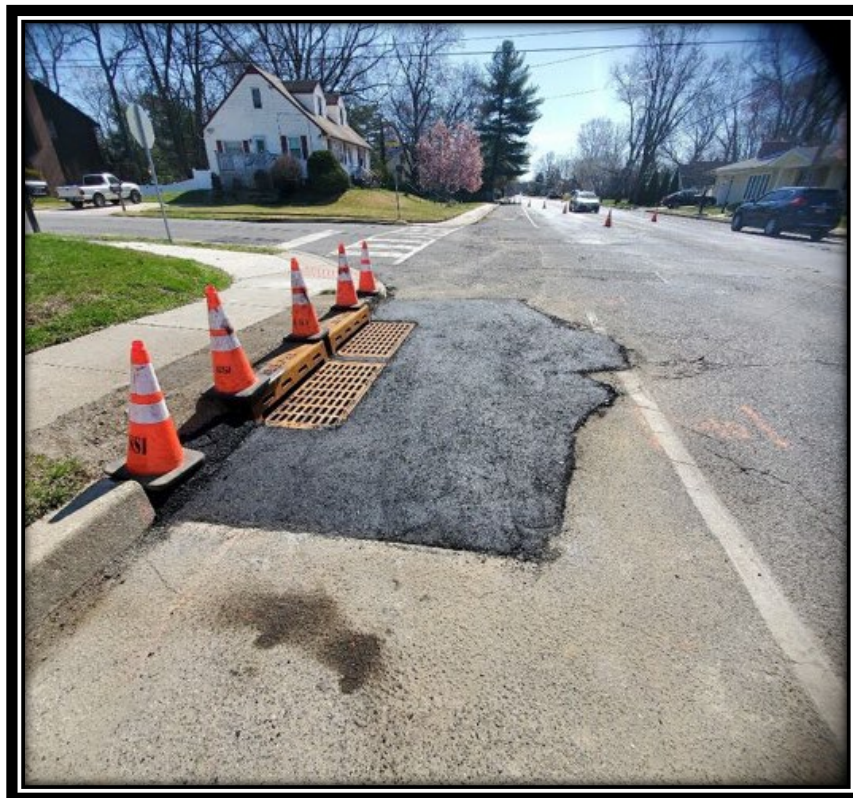
Figure: 3 – HMA restoration in front of newly installed Type Double B Inlet along the northbound lane at the intersection with Cedar Avenue
