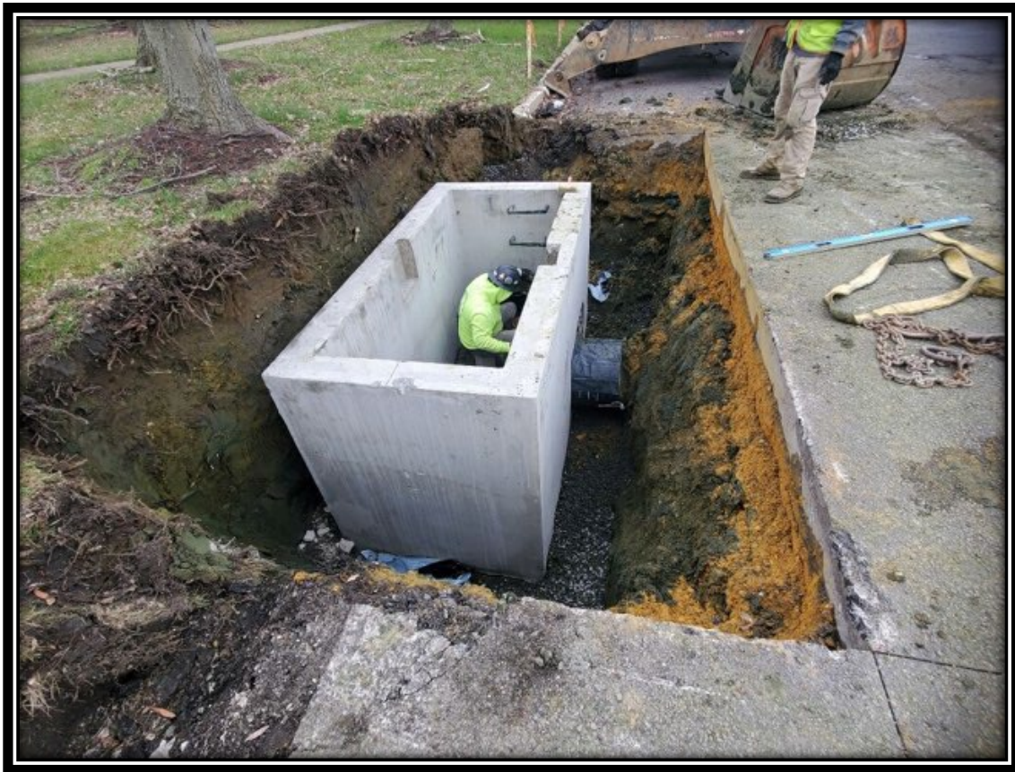
Figure: 1 – Installation of Type Double B Inlet along the northbound lane between Somerdale Road and Laurel Road
