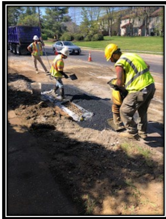
Figure: 3 – HMA restoration in front of newly installed Double B Inlet along the eastbound lane between DaCosta Drive and Kings Highway
