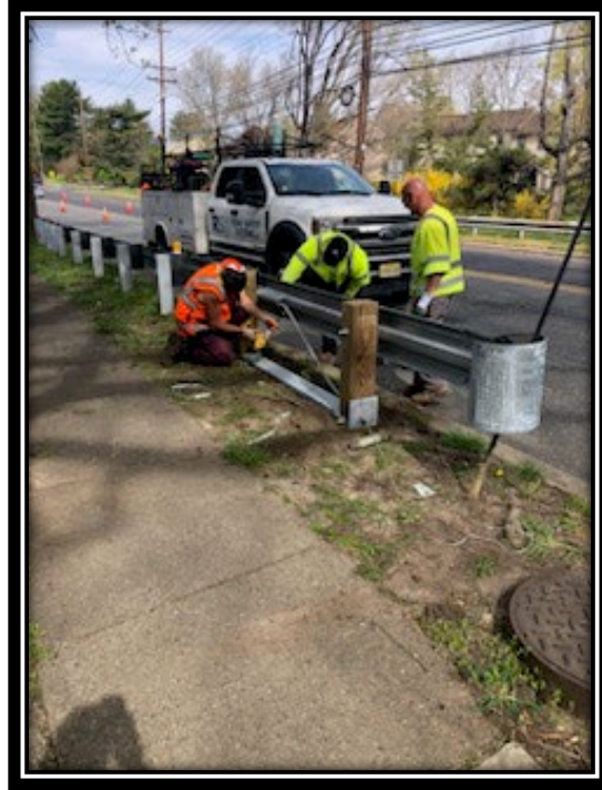
Figure: 2 – Installation of Beam Guide Rail along the eastbound lane between Crofton Commons and DaCosta Drive
