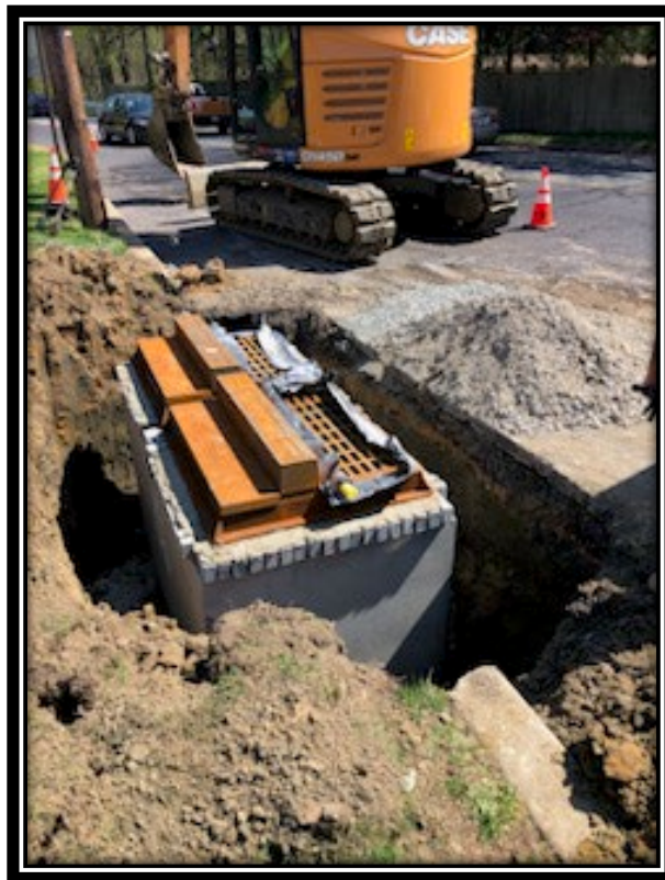
Figure: 1 – Installation of Double B Inlet along the eastbound lane between DaCosta Drive and Kings Highway
