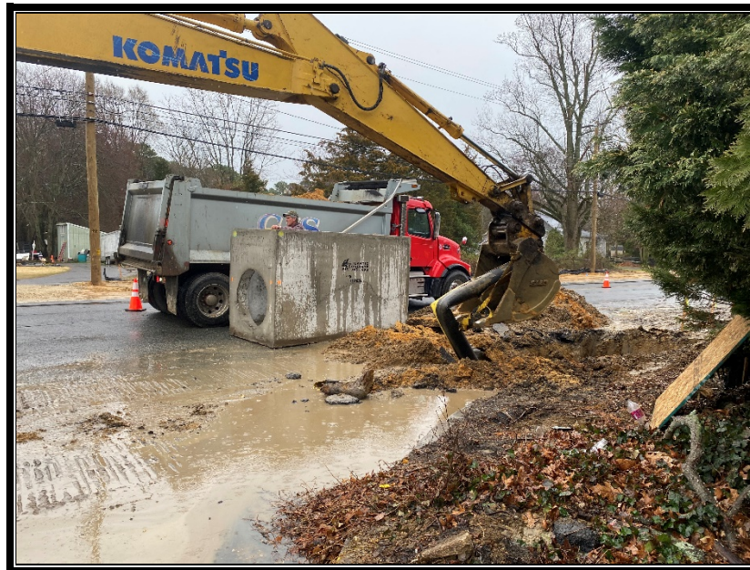
Figure 3: P&A Construction installing precast concrete Inlet Type "Double B" and removal of old, existing South Jersey Gas Company gas main.
