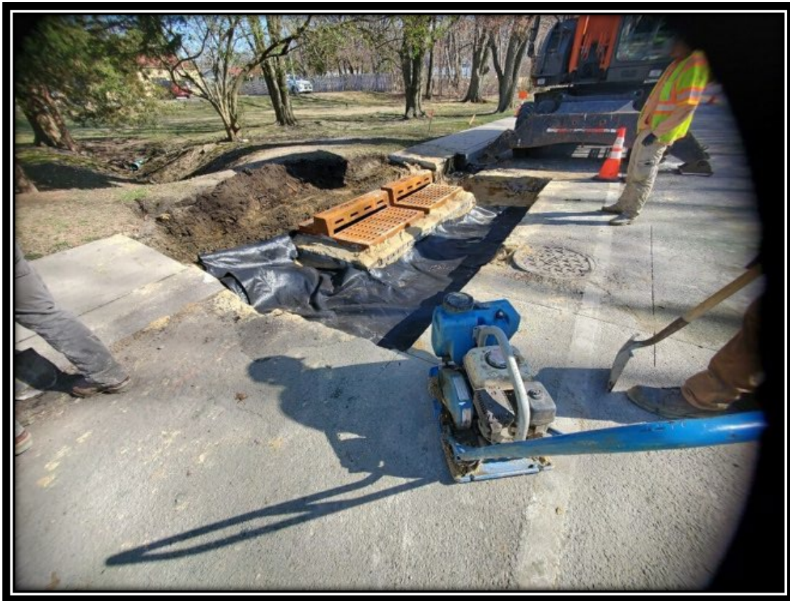
Figure: 1 – Installation of Type Double B Inlet along the northbound lane between Britton Place and Elm Avenue
