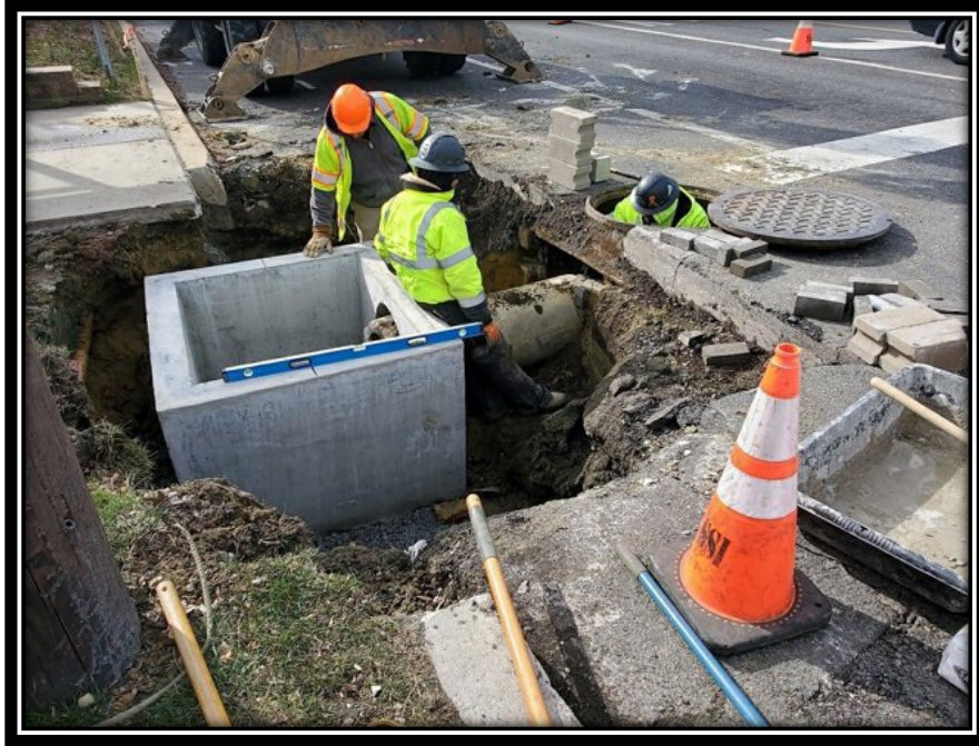
Figure: 2 – Installation of Type B Inlet along the northbound lane at the intersection with Somerdale Road
