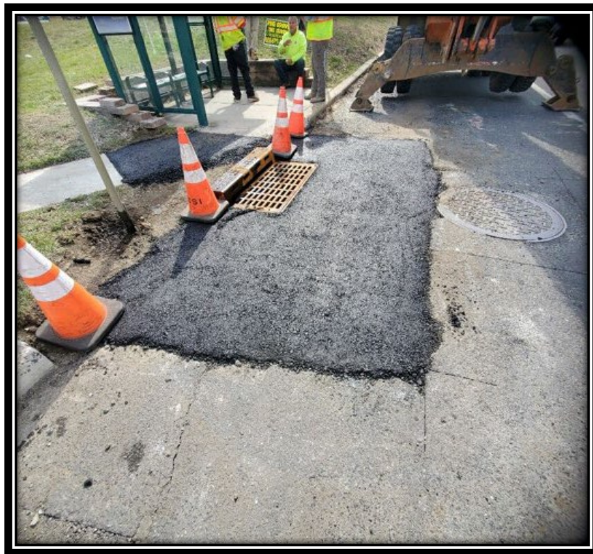
Figure: 3 – HMA restoration in front of newly installed Type B Inlet along the northbound lane at the intersection with Somerdale Road
