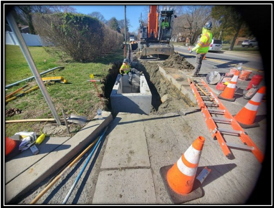
Figure: 1 – Installation of Type Double B Inlet along the southbound lane at the intersection with Maple Avenue
