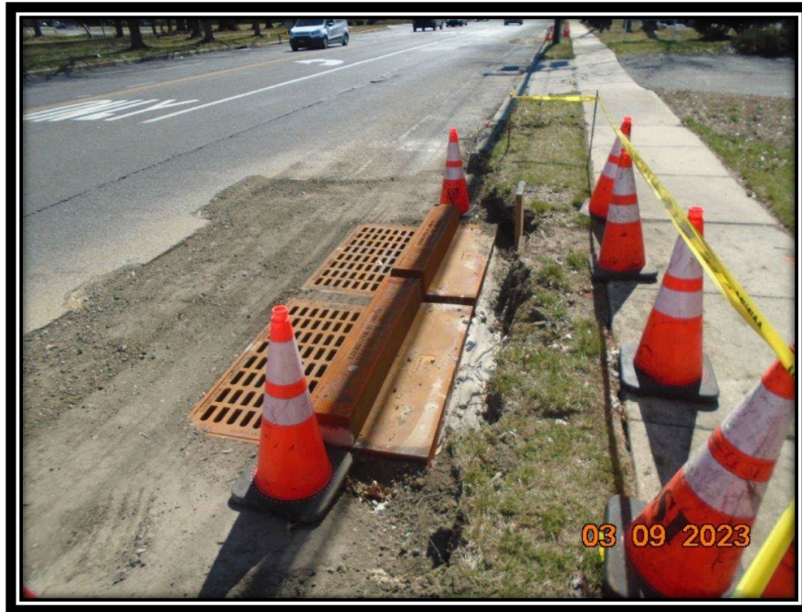
Figure: 2 – Installation of Type Double B Inlet along the southbound lane between Laurel Road and Britton Place
