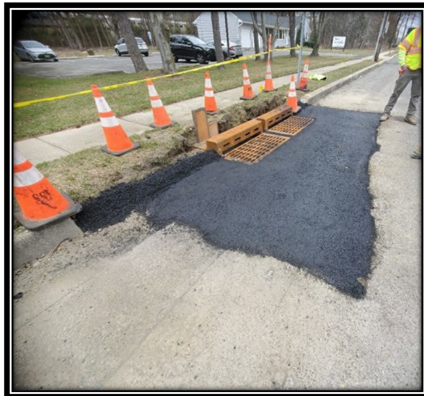
Figure: 3 – HMA restoration in front of newly installed Type Double B Inlet along the southbound lane between Laurel Road and Britton Place
