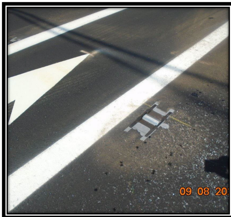
Figure: 3 – Installation of raised pavement markings along the northbound lane between Cedar Avenue and Britton Place
