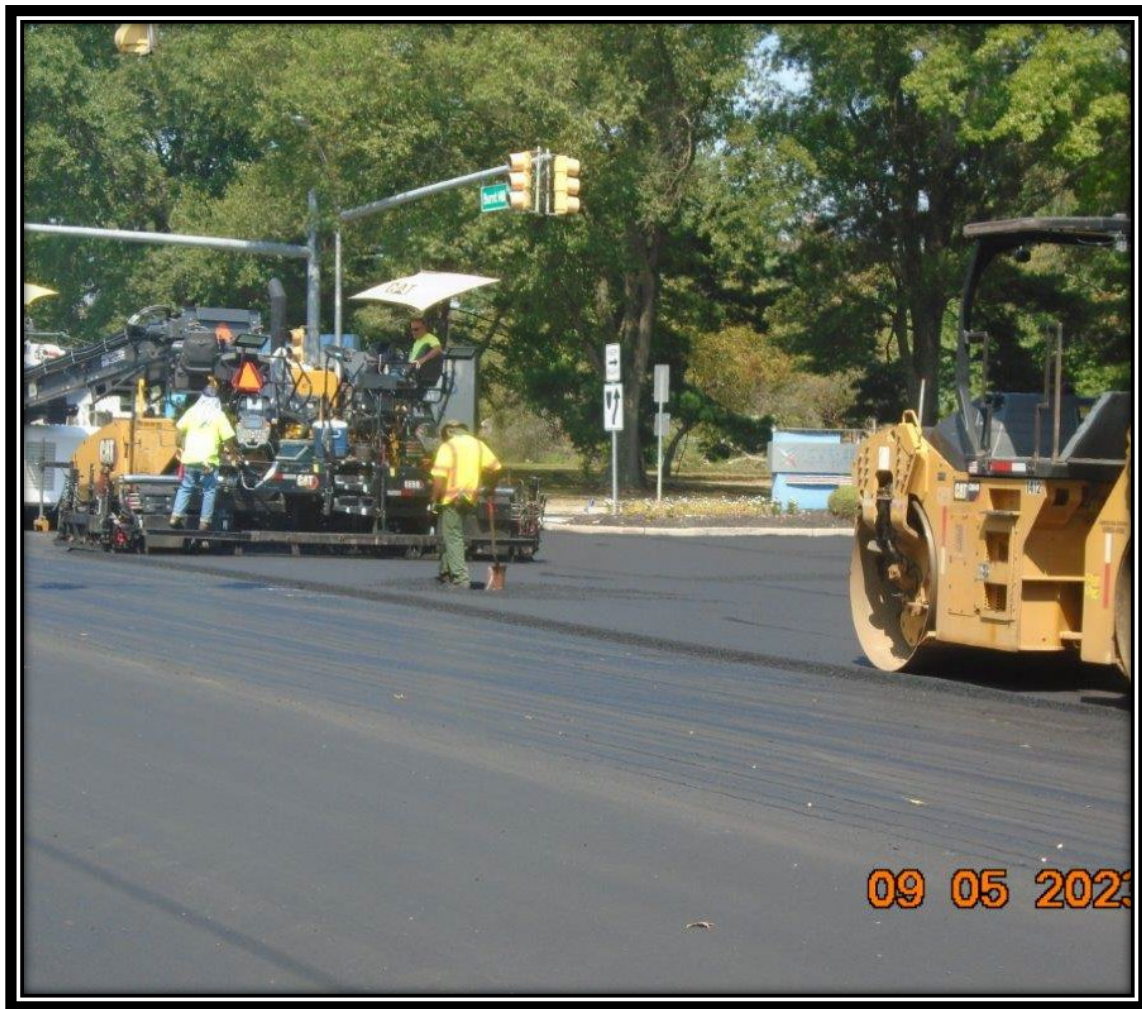
Figure: 1 – Installation of HMA 12.5M64 Surface Course along the northbound lane at the intersection with Laurel Road
