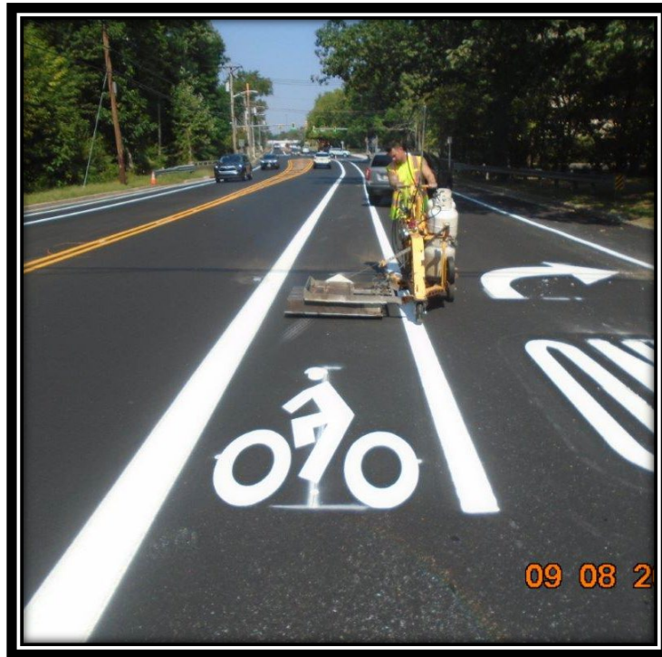
Figure: 2 – Installation of thermoplastic traffic striping and markings along the northbound lane between Cedar Avenue and Britton Place
