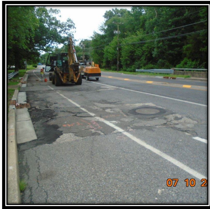
Figure: 2 – Resetting of an existing sanitary sewer manhole along the northbound lane between Maple Avenue and Britton Place
