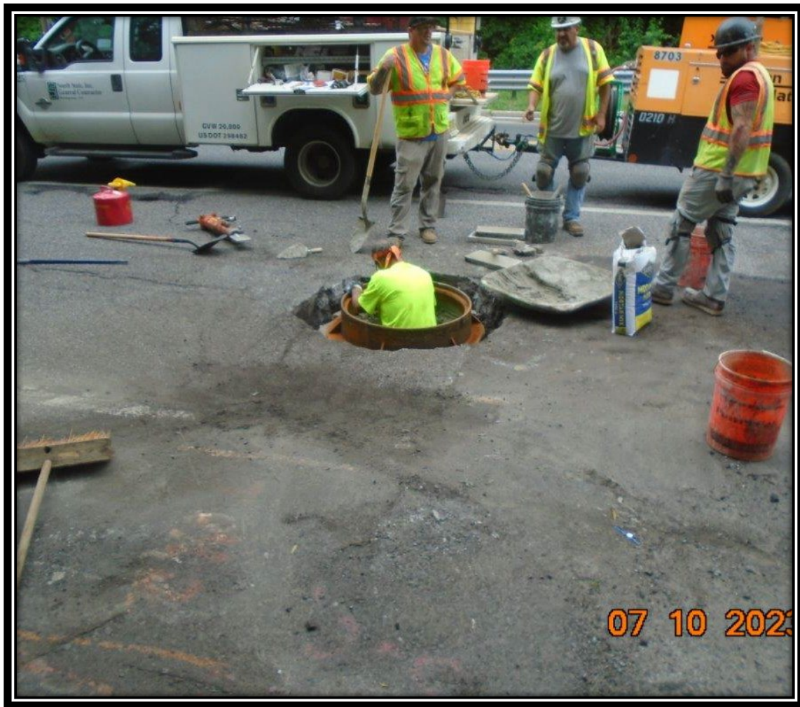
Figure: 1 – Resetting of an existing sanitary sewer manhole along the northbound lane between Maple Avenue and Britton Place
