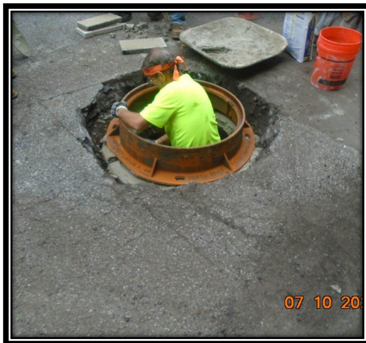
Figure: 3 – Resetting of an existing sanitary sewer manhole along the northbound lane between Maple Avenue and Britton Place
