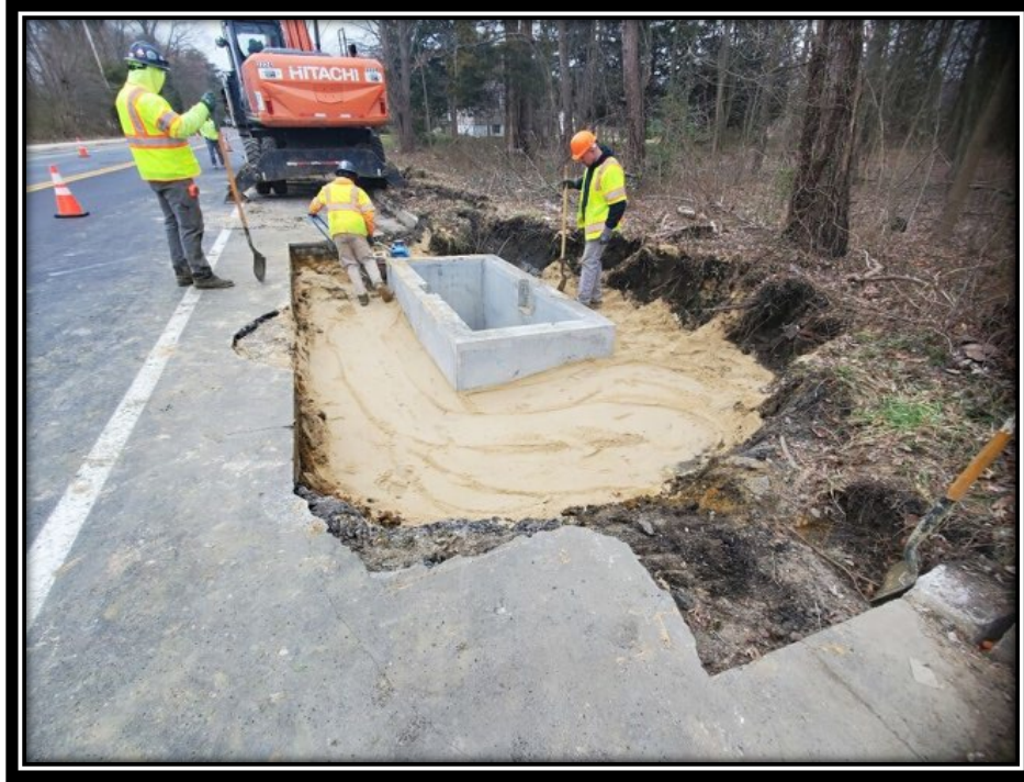
Figure: 2 – Installation of Type Double B Inlet along the southbound lane between Britton Place and Elm Avenue
