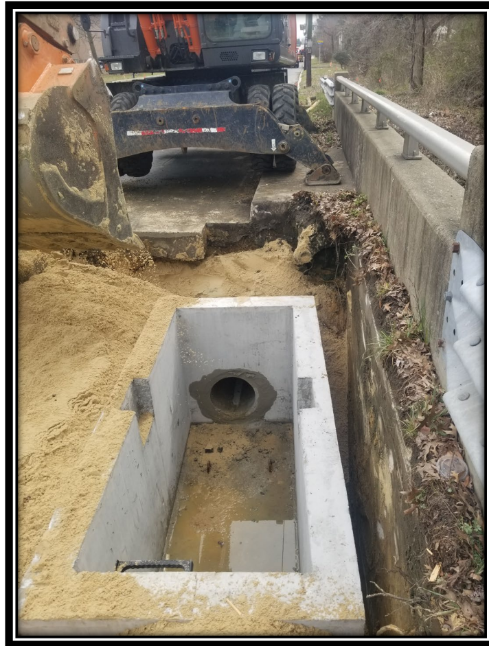
Figure: 1 – Installation of Type Double B Inlet along the southbound lane between Laurel Road and Britton Place
