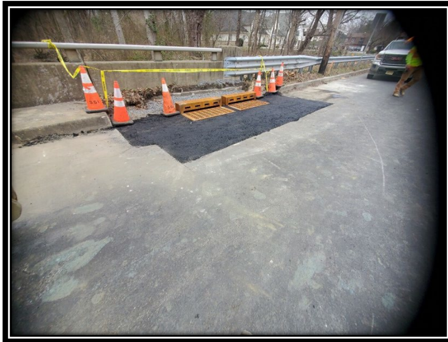
Figure: 3 – HMA restoration in front of newly installed Type Double B Inlet along the southbound lane between Laurel Road and Britton Place
