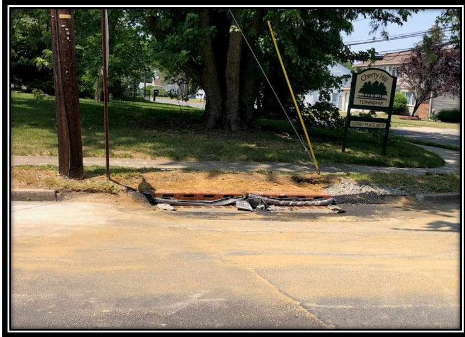
Figure: 2 – Installation of Double B inlet at the intersection with Surrey Road
