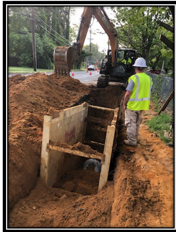
Figure: 3 – Installation of 18" RCP along the eastbound lane between Friendship Lane and Millstream Drive
