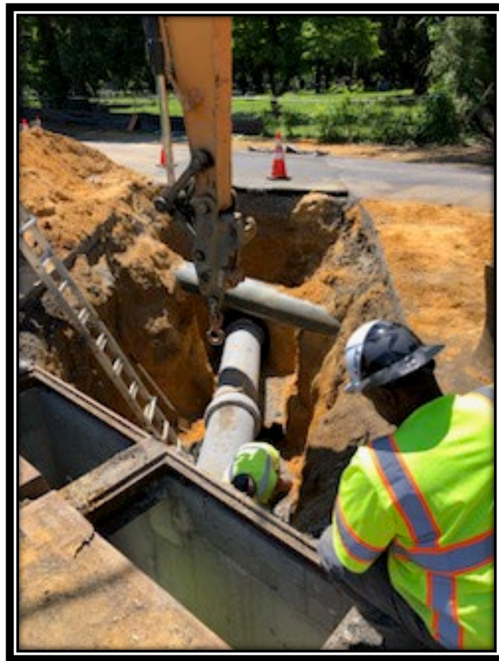
Figure: 1 – Connection of 18” RCP storm sewer crossing at the intersection with Millstream Drive
