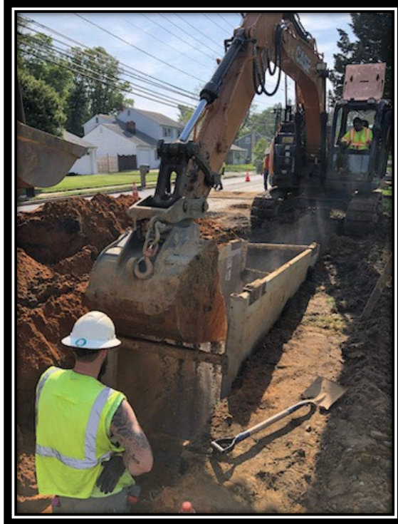
Figure: 2 – Setting of trench box for the installation of 18” RCP storm sewer along the eastbound lane between Millstream Drive and Friendship Lane
