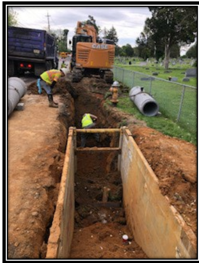
Figure: 1 – Connection of 18” RCP along the eastbound lane between Millstream Drive and Friendship Lane
