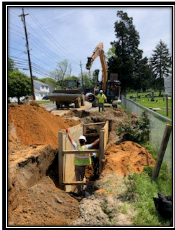
Figure: 3 – Connection of 18” RCP along the eastbound lane between Millstream Drive and Friendship Lane
