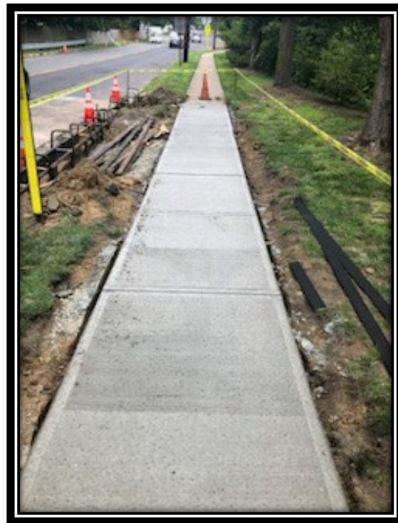
Figure: 3 – Installation of concrete sidewalk along the westbound lane between the Thomas Paine Elementary School and King's Croft Drive
