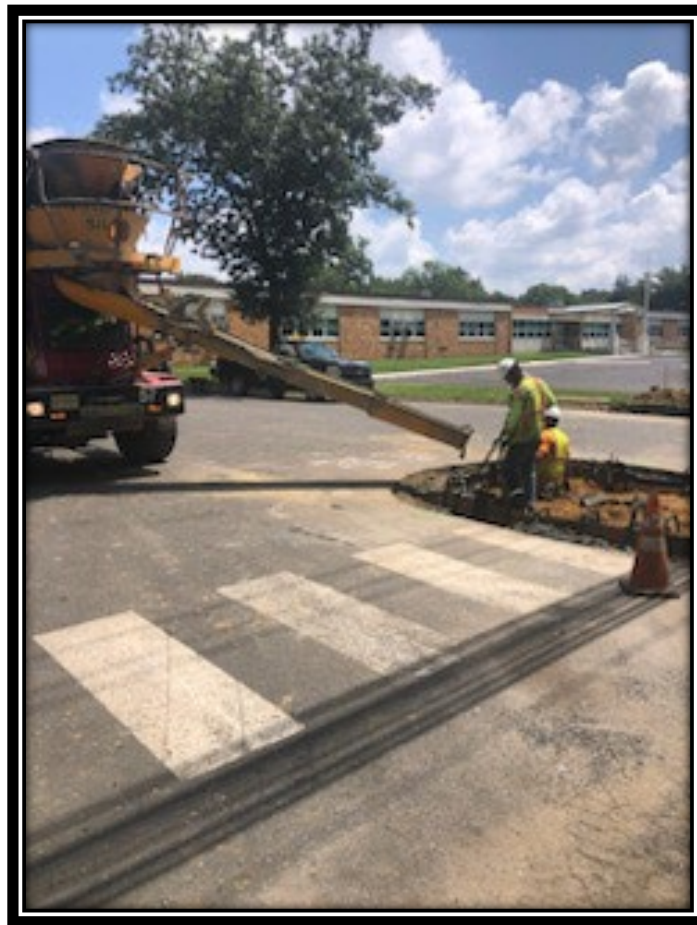
Figure: 1 – Installation of concrete vertical curb along the westbound lane at the entrance to the Thomas Paine Elementary School
