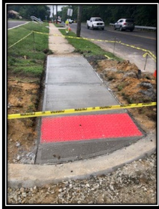
Figure: 2 – Installation of ADA ramp and concrete sidewalk along the westbound lane in front of the Thomas Paine Elementary School
