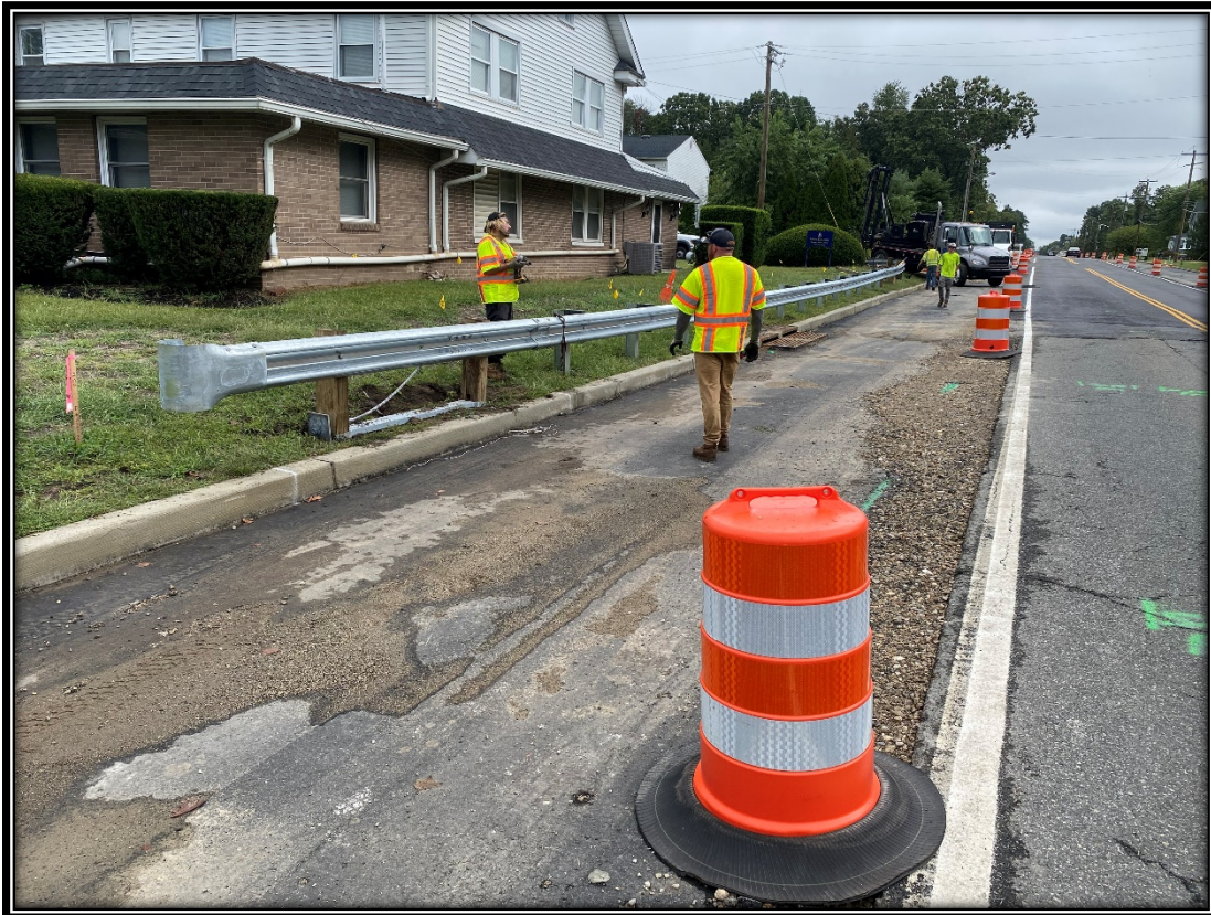
Figure: RSS Roadway Safety Systems, LLC installing guide rail and end treatments.
