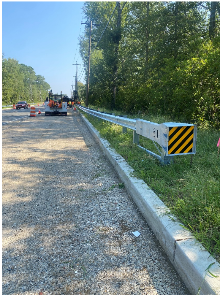
Figure: RSS Roadway Safety Systems, LLC installing guide rail and end treatments.
