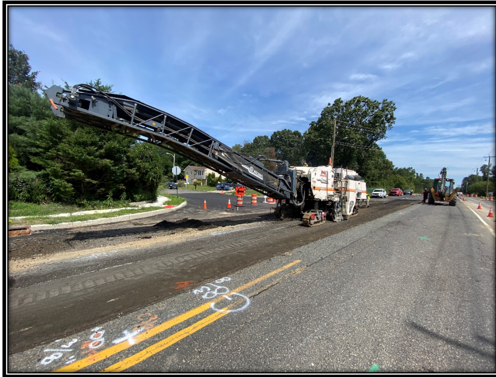
Figure: P&A Construction continues to mill the existing roadway in order to construct the new roadway
