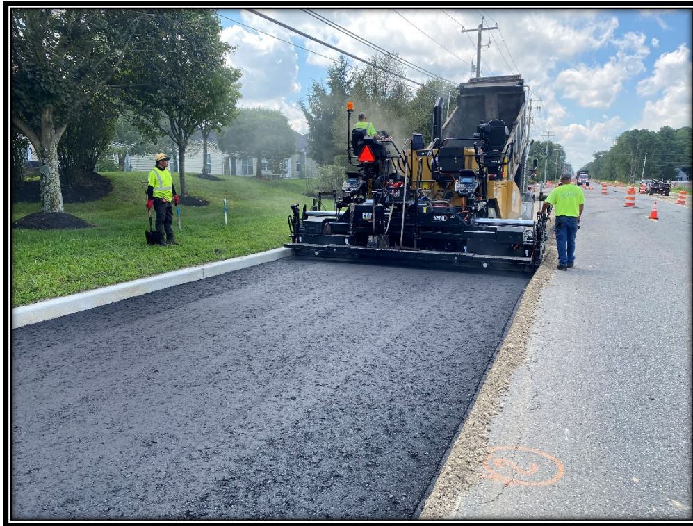
Figure: P&A Construction continues to install the hot mix asphalt, using their brand new CAT AP 1055.
