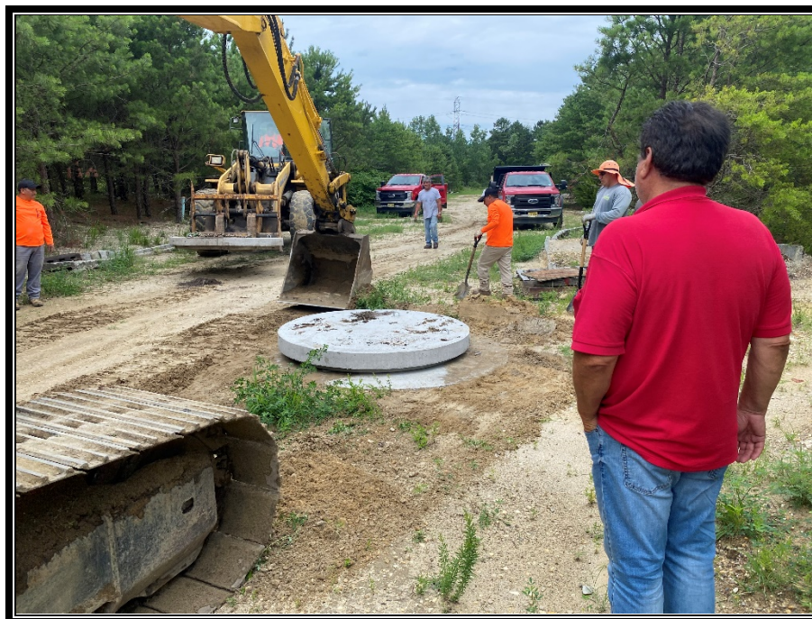
Figure 3: P&A Construction installing pre-cast concrete slabs on manholes in off-site drainage easement.
