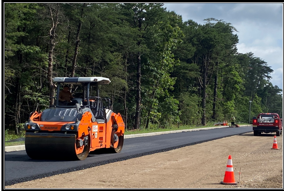
Figure 2: P&A Construction started started to install the hot mix asphalt base course.
