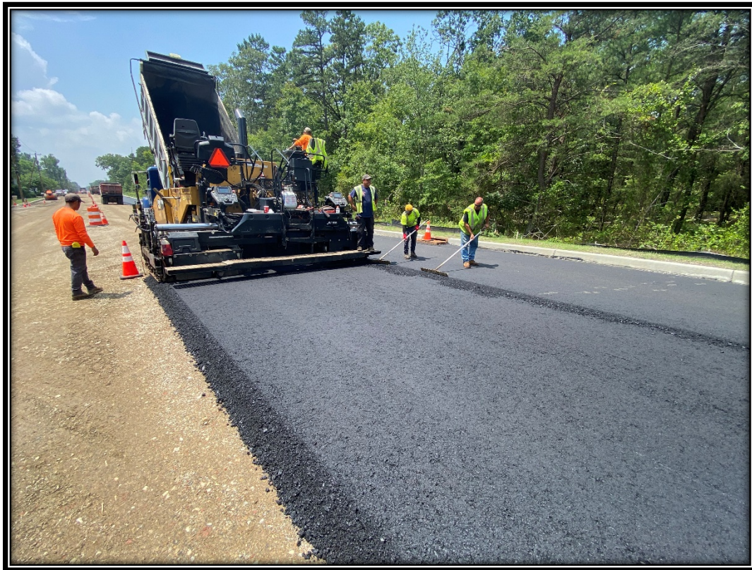
Figure: P&A Construction started to install the hot mix asphalt base course.
