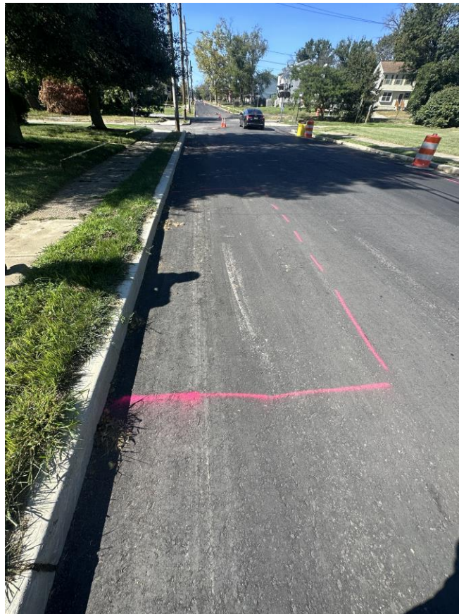
Figure 2. Areas in need of base repair prior to placement of HMA surface course were marked out in the field during proof roll.
