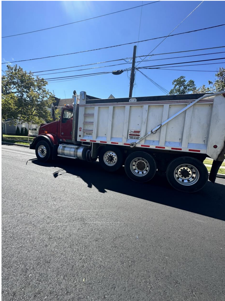
Figure 1. The contractor, South State, performed a proof roll of the base paving to determine which areas are in need of repair prior to installation of HMA surface course.
