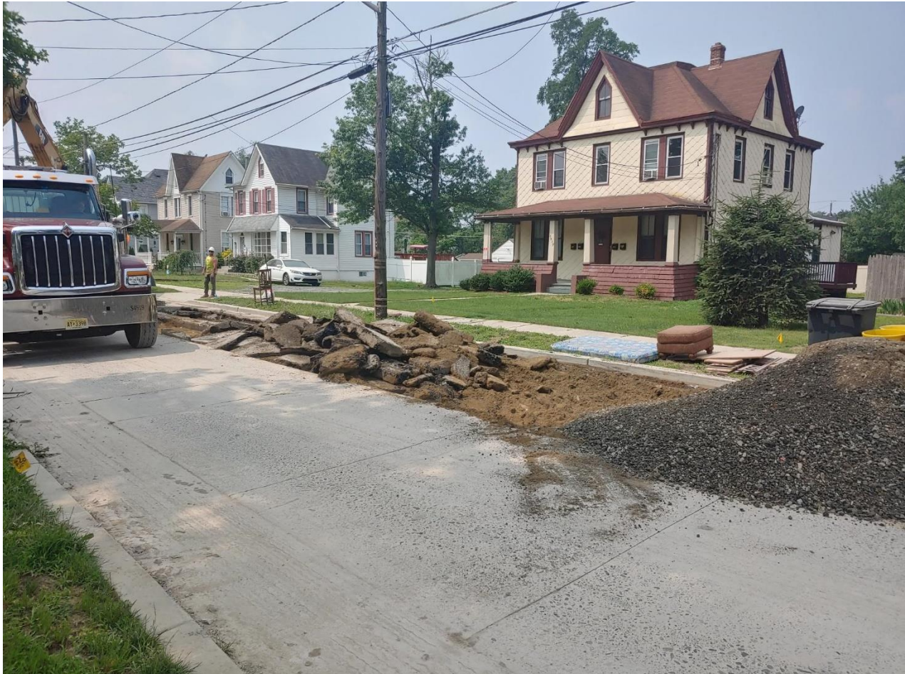
Figure 1. The contractor, South State, continued work on Union Avenue by removing concrete roadway.
