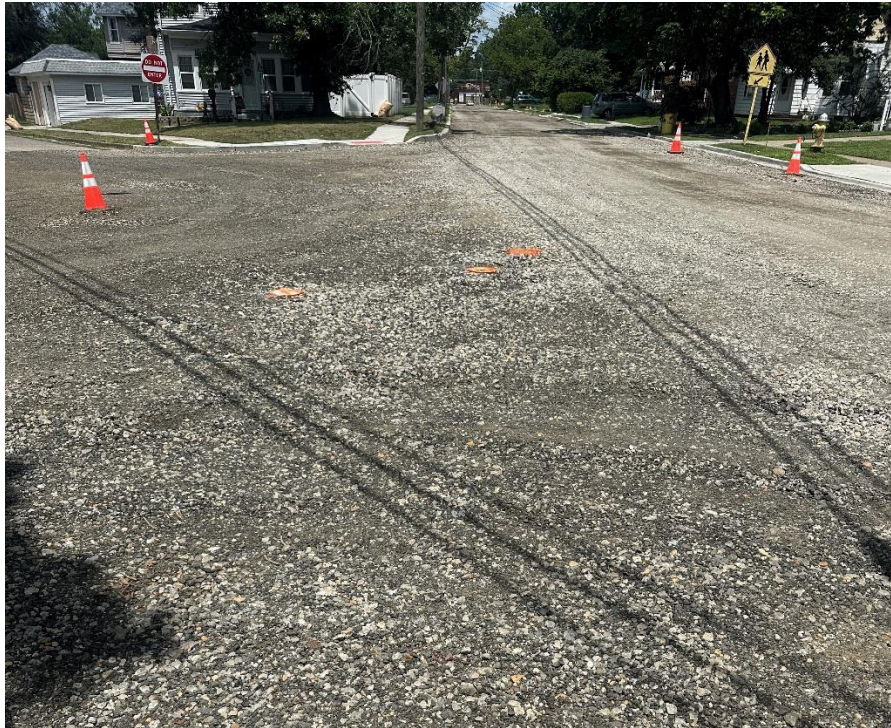
Figure 2. The contractor, South State, placed and compacted DGA within the areas of concrete road removal to act as a temporary road condition prior to FDR (Full Depth Reclamation) and Final Paving.
