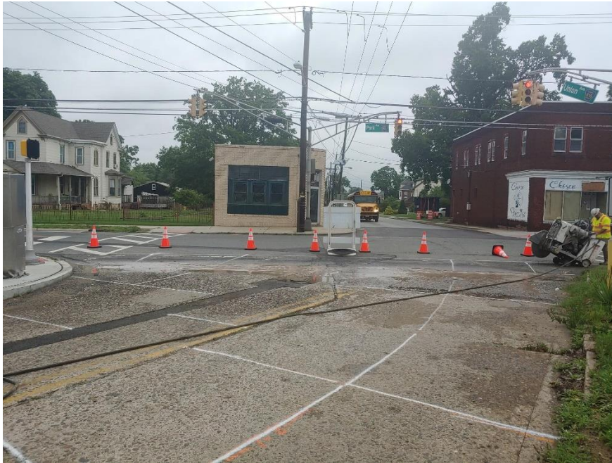
Figure 1. The contractor, South State, resumed work on Union Avenue following the PSE&G work/Winter Shutdown and began sawcutting road in order to remove existing concrete slabs.
