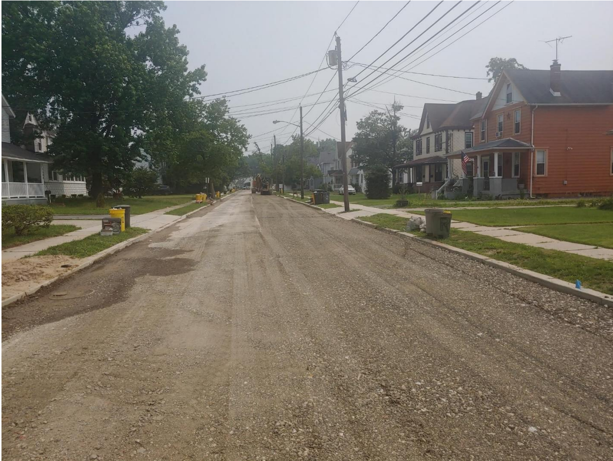
Figure 3. The contractor, South State, spread and compacted the DGA within Union Avenue to act as a temporary condition for the road prior to FDR (Full Depth Reclamation) and Final Paving.
