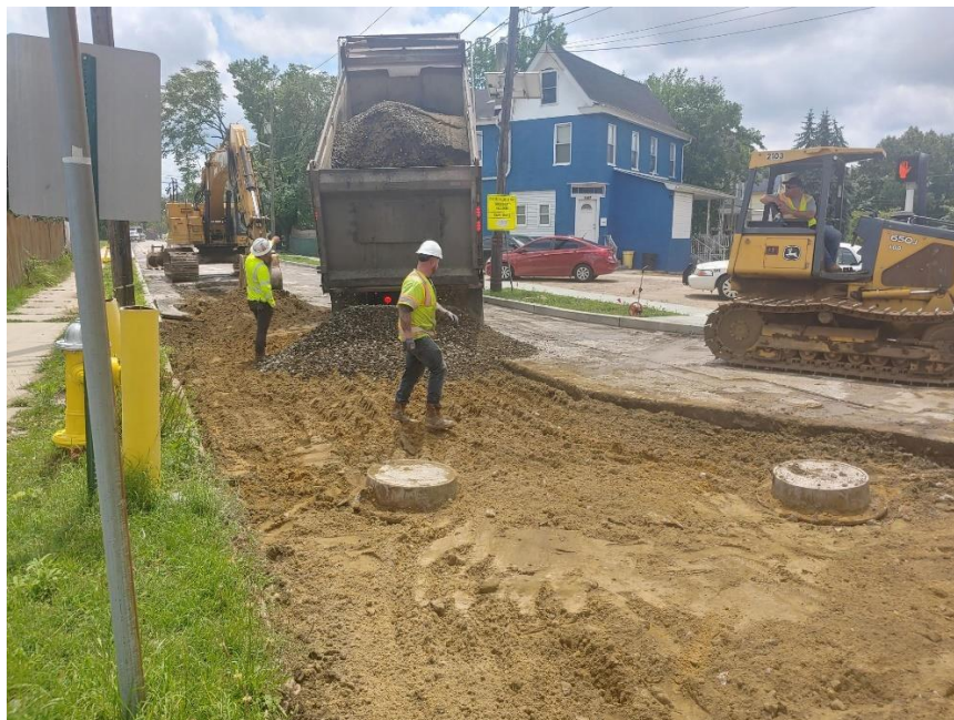
Figure 2. The contractor, South State, placed DGA within the areas of concrete road removal.
